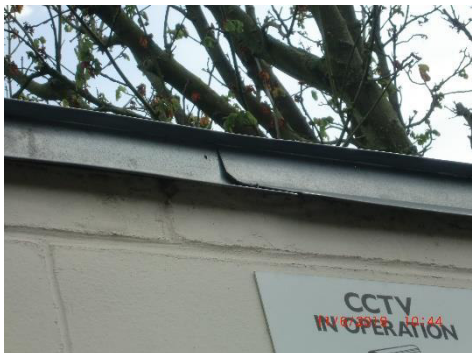
Photo 5: Partially lifted lead flashing in southern corner
