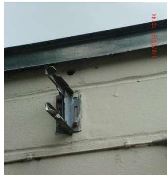
Photo 5: Small hole in wall in southern corner
