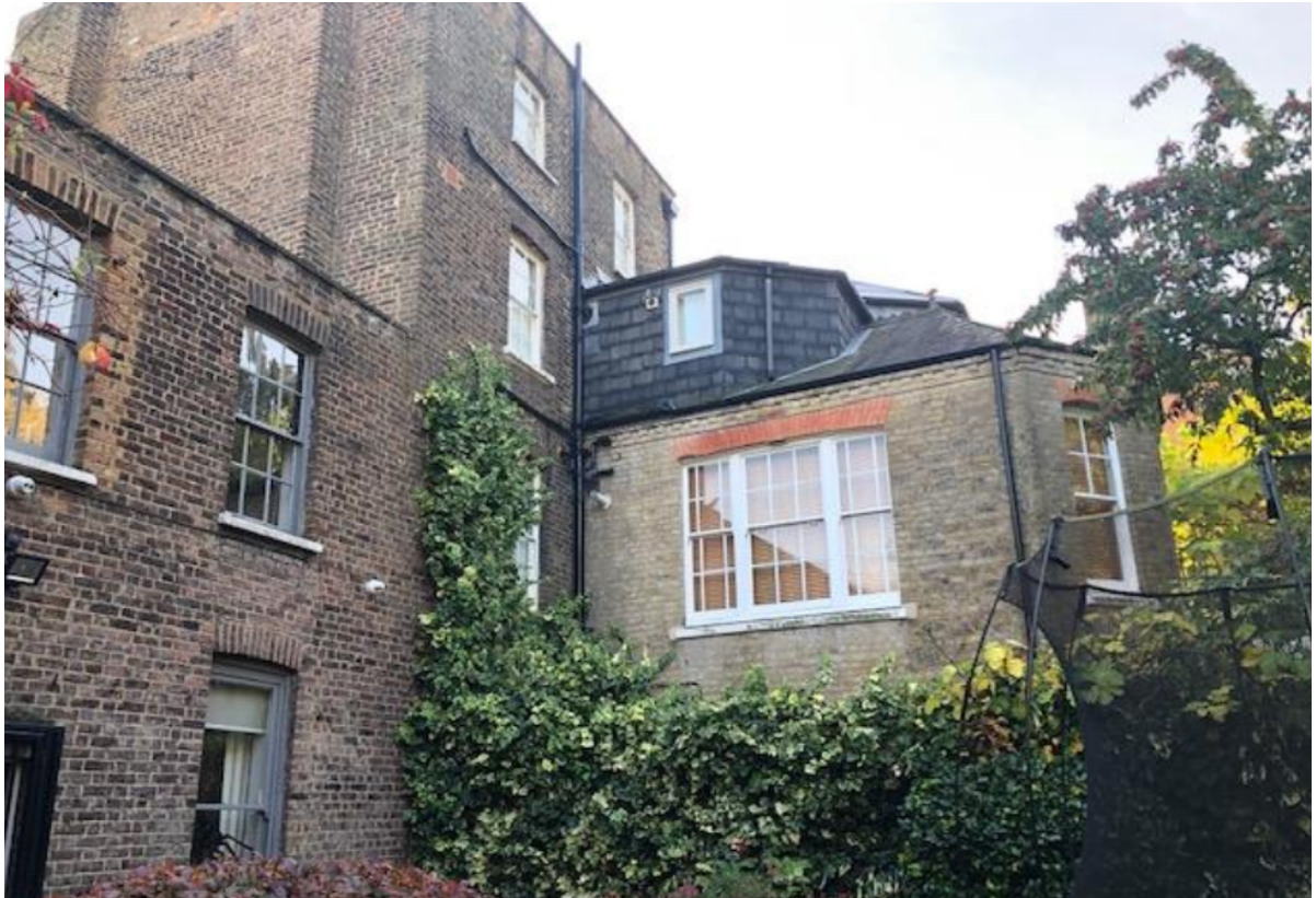
3) Rear extension of adjoining no.7 (taken from the rear garden of the application site)
