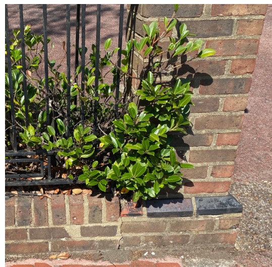
View of existing wall base showing cracking
