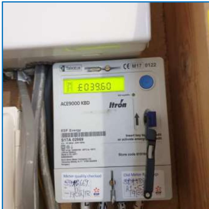
Flat 9 – Electricity pre-pay meter
