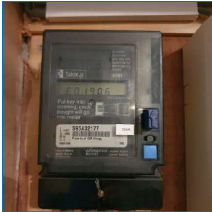
Flat 10 – Electricity pre-pay meter
