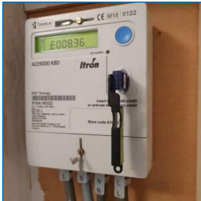
Flat 2 – Electricity pre-pay meter
