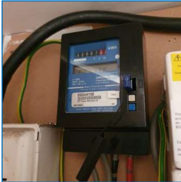
Flat 5 – Electricity pre-pay meter
