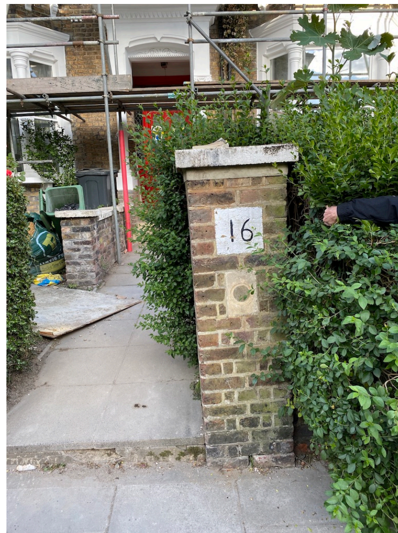
Central piers are not straight and in need of renovation
