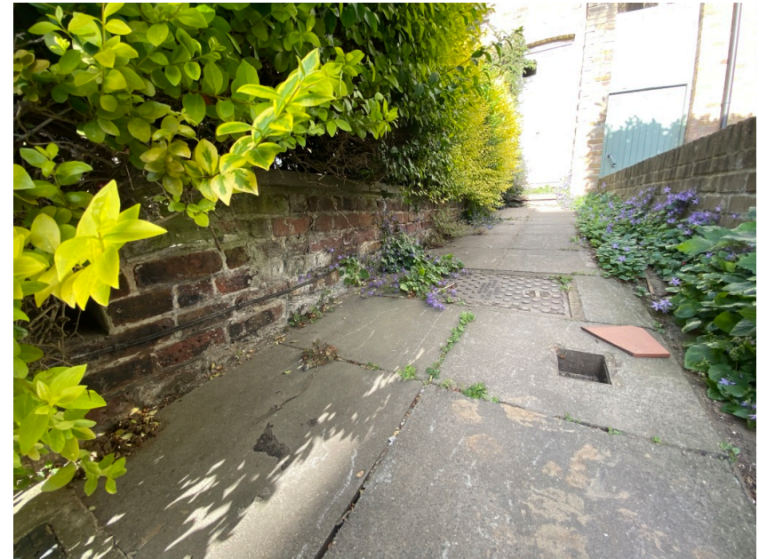
Concrete pavers to side entrance and damaged dwarf wall
