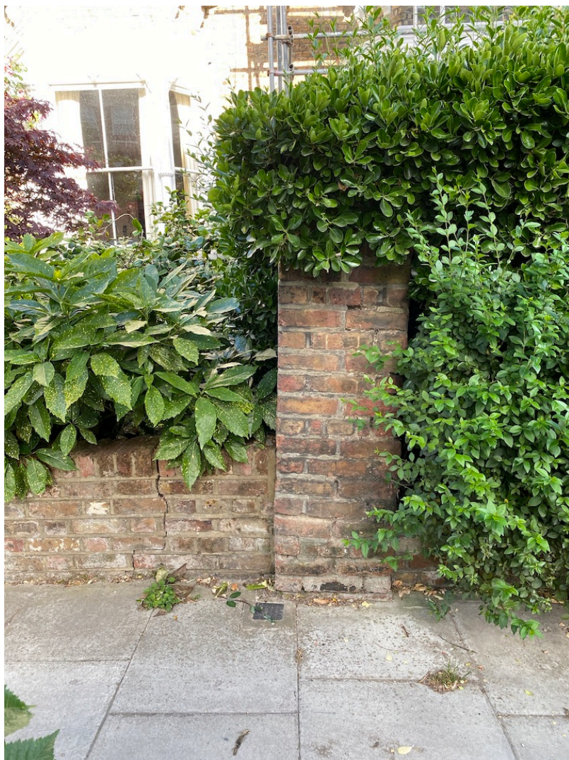
Left hand side pier with cracked dwarf wall
