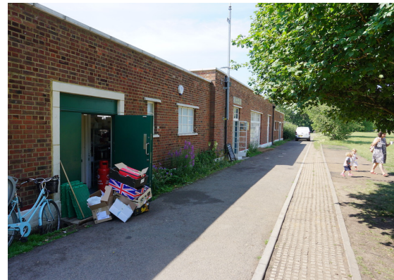
The rear elevation is plain and functional. It has recently been altered to allow the café to open onto the park.
