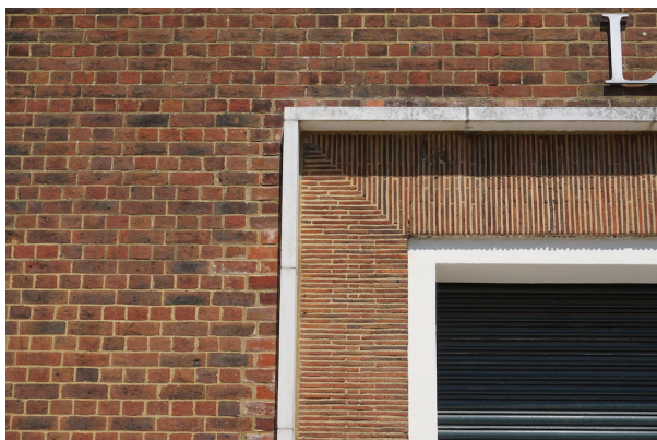
English Bond brickwork and fine tile creasing are a subtle adaptation to vernacular traditions.
