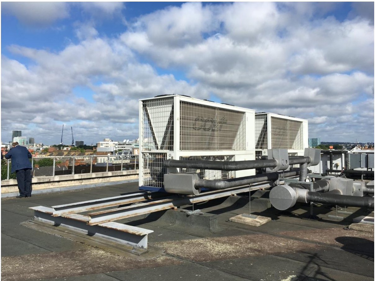
Existing Rooftop Building Services Plant
