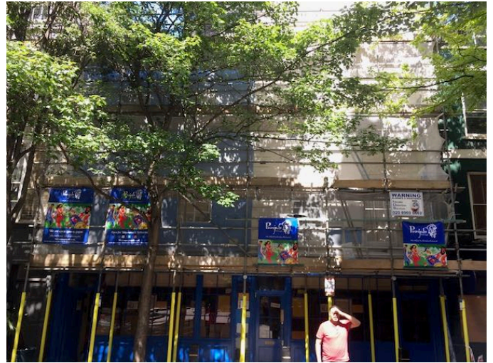
Front elevation of 80 and *2 Neal Street showing the first coat of paint on No 82 Neal Street
