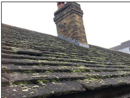
Figure 6: Lifted tile on gable roof
