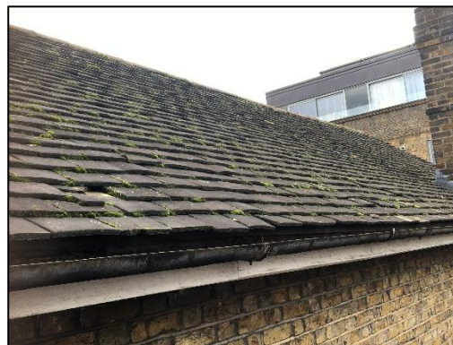
Figure 7: Missing tile on gable roof
