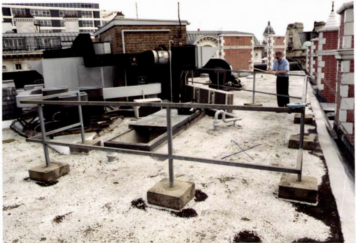
ROOF EXISTING A/C PLANT ↗
