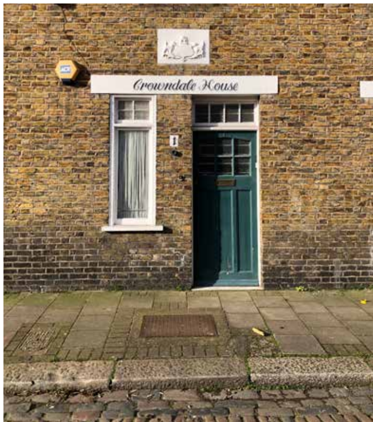
photo of existing cobbles and paving showing weathered brickwork of exg. building
