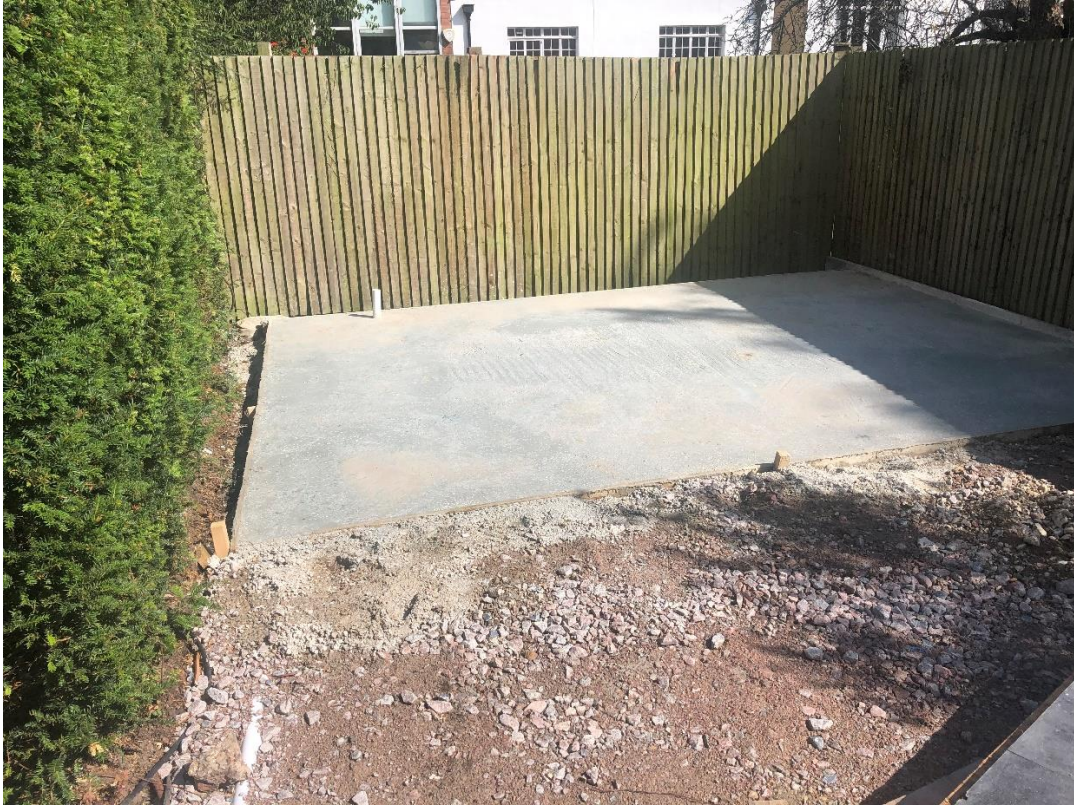
43 Ferncroft Avenue, London NW3 – location of proposed garden room at rear of rear garden, bordered by existing hedges and timber fencing
