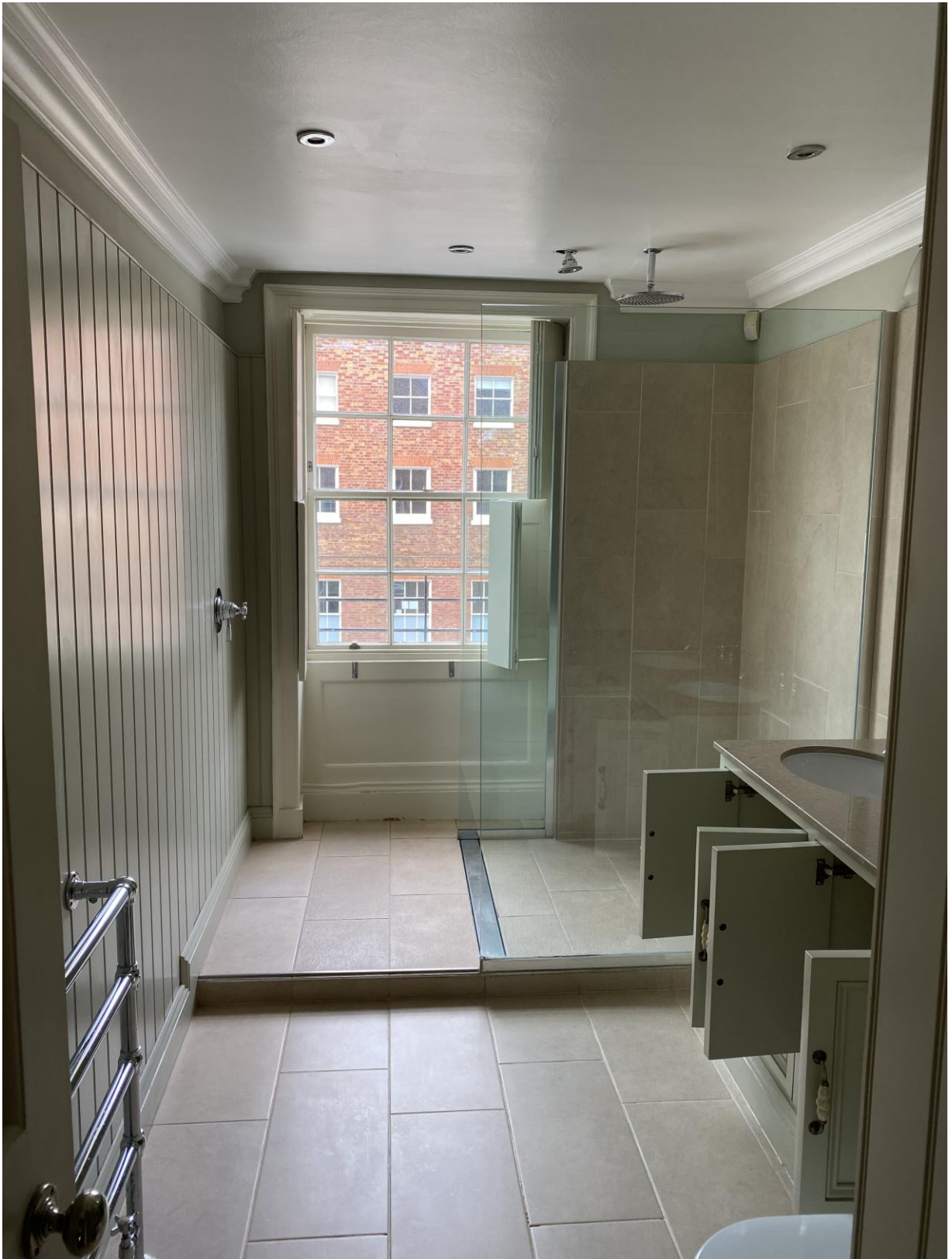
4.5 Second floor bathroom. Lath and plaster ceiling; painted plaster walls; moulded plaster cornice; 6/6 double hung sliding sash window; ovolo moulded panelled shutters, soffit and recess down to floor; ogee moulded architraves; ogee moulded skirting boards; ceramic tile floor.
