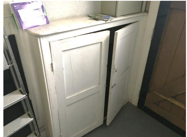
Photo 12. Electrical cupboard within communal entrance hall
