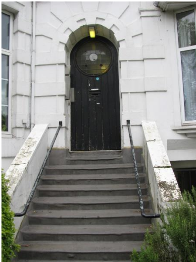
Photo 11. No. 5 Oak Court - communal front entrance steps
