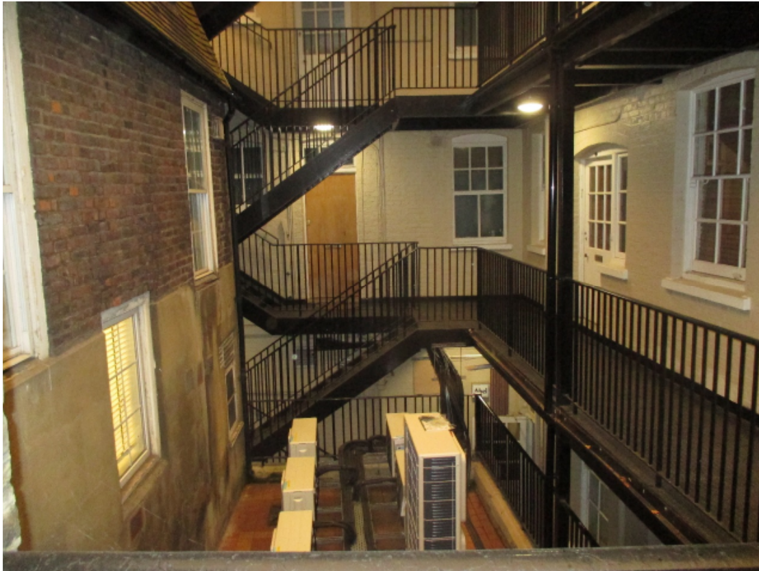
1. Taken from 1 st floor level showing existing a/c units within courtyard
