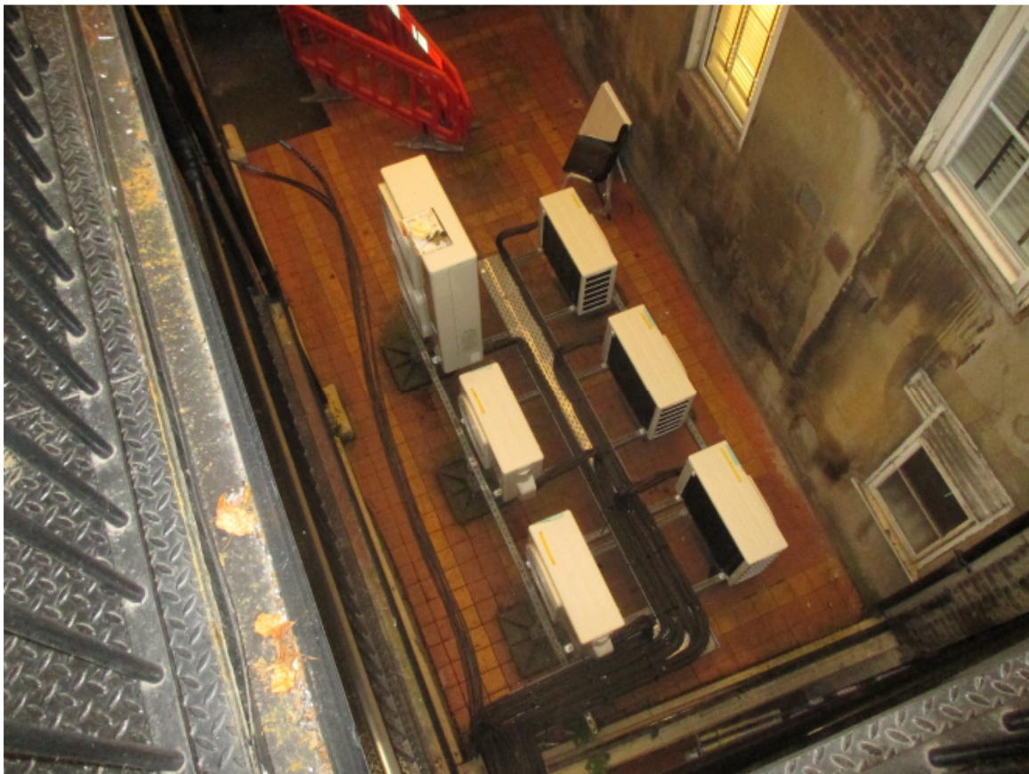
2. Taken from 2 nd floor showing existing a/c units with rear of bank
