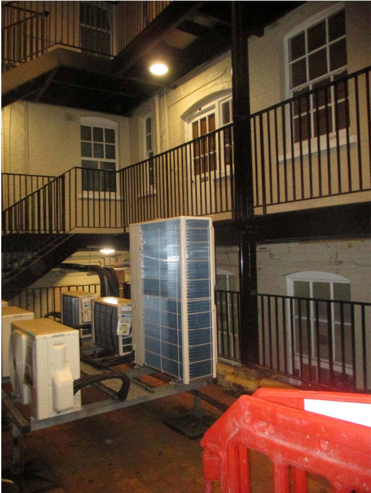
3. Air conditioning units showing nearest window
