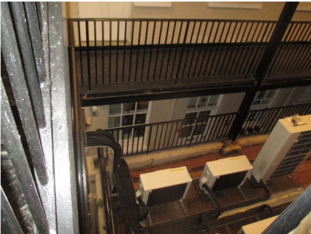
5. View looking down on a/c units
