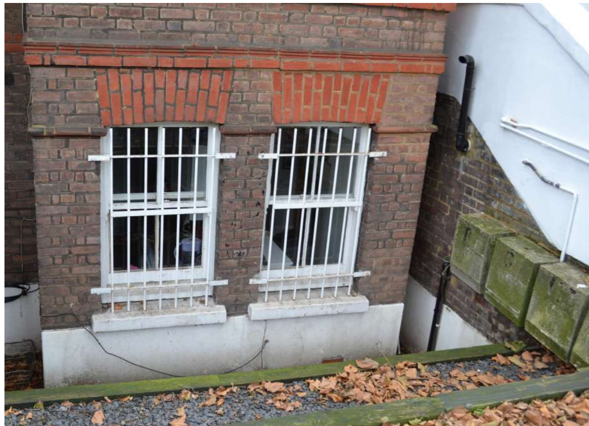
▲ Fig 25. Example of existing sash windows on front elevation with security bars
