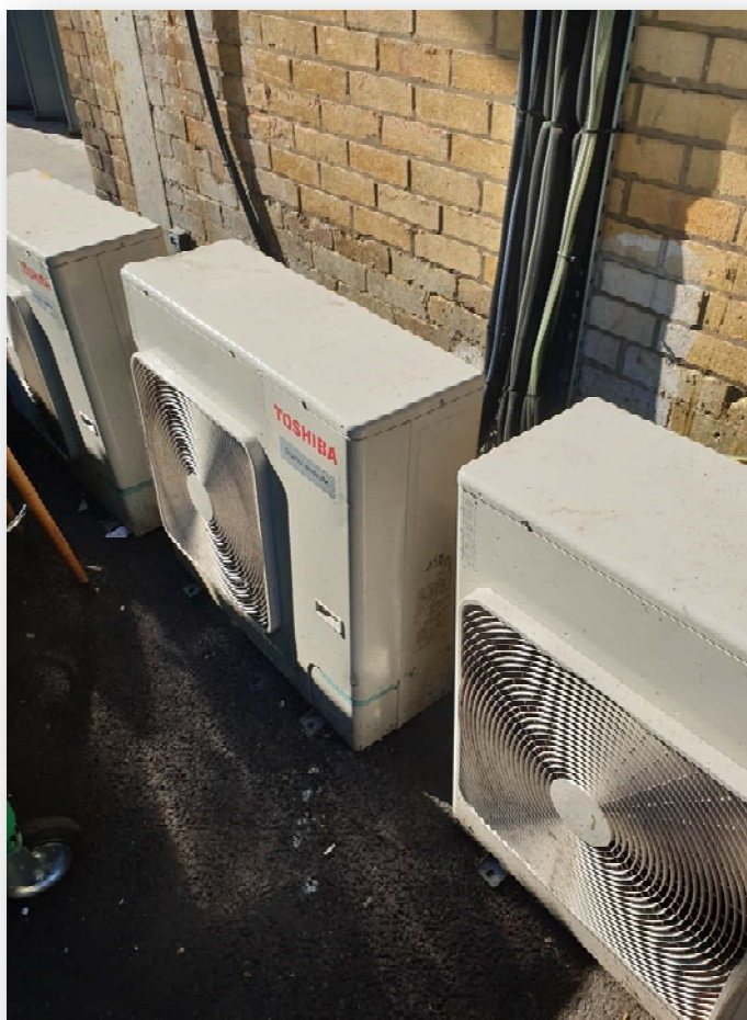
FIGURE 1: Toshiba AC units, Deliveroo Swiss Cottage
