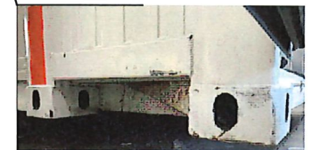
Hoist point frame
