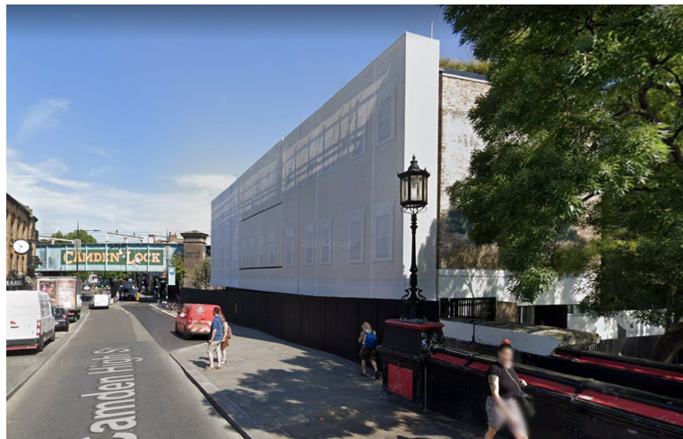
Figure 5 - Three storey building being constructed to the opposite side of the lock
