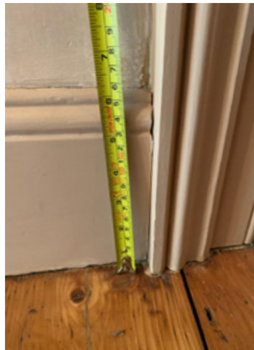
existing view 3 showing original skirting & architraving to lobby/landing with original floor boards
