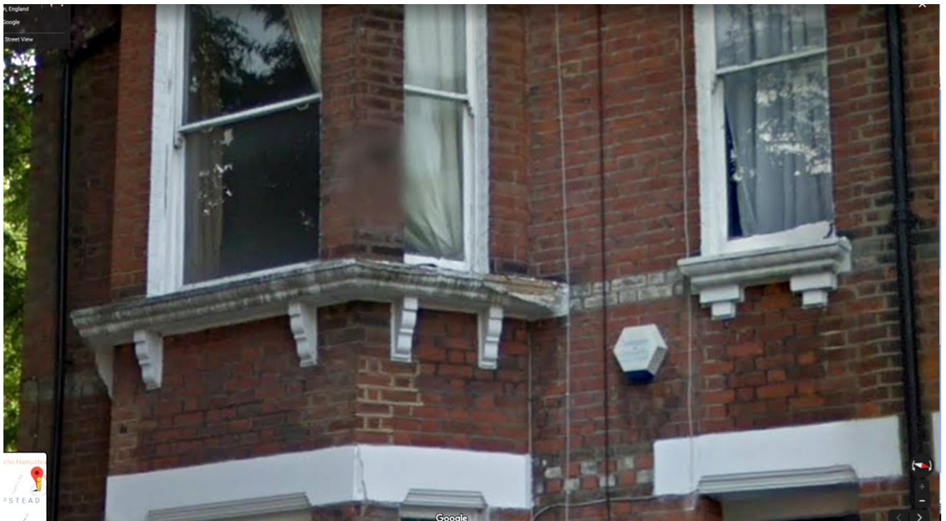
May 2012 showing many different mortar repairs over the years
