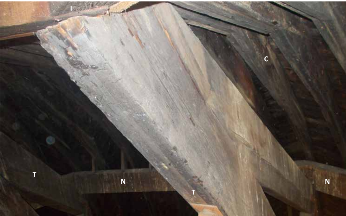
Figure 18: Another view of the tie beam end of truss at the apex (2019) © H&R
