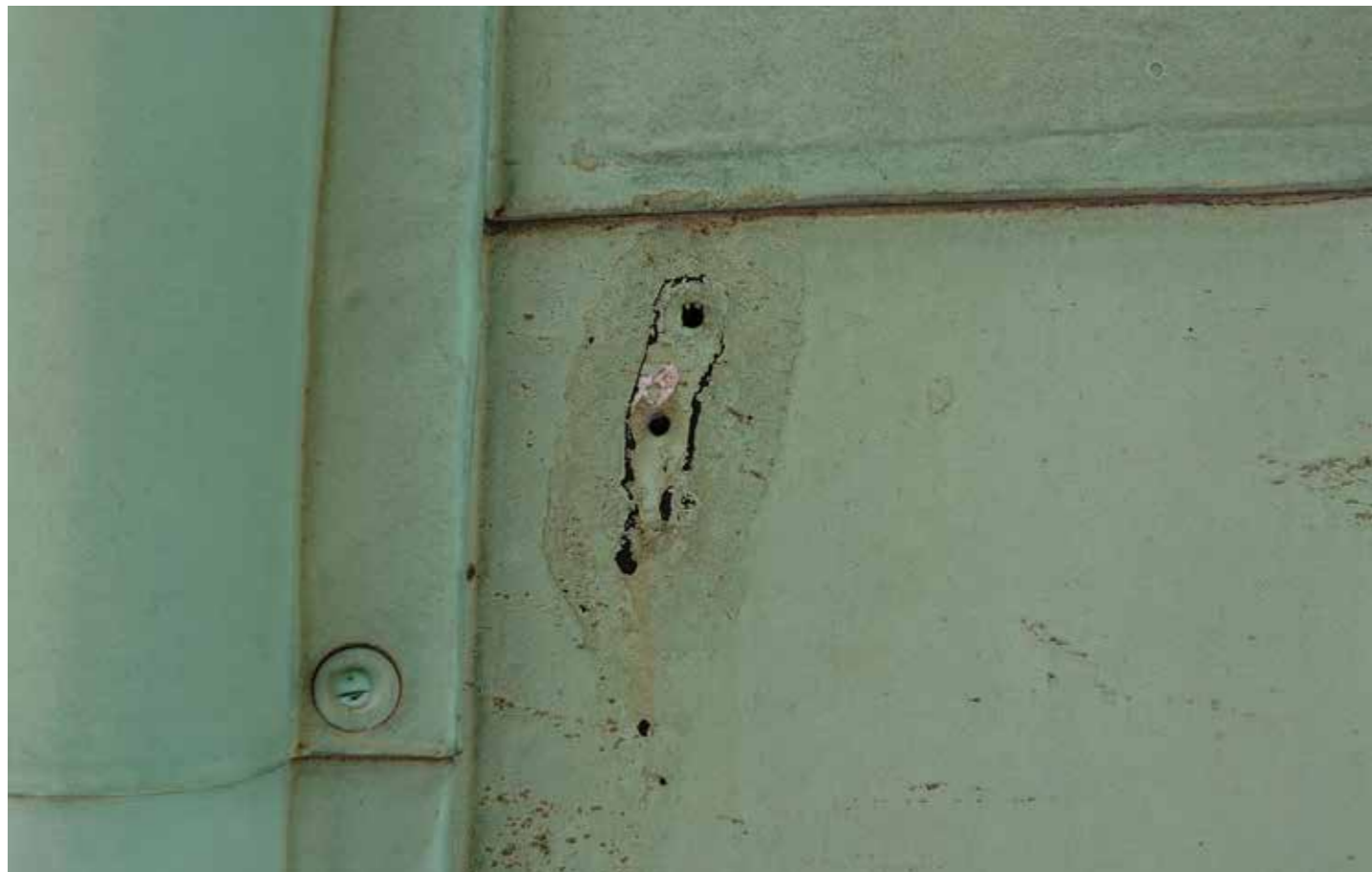
Figure 24: Exterior copper roof cladding detail and damage (2019) © H&R
