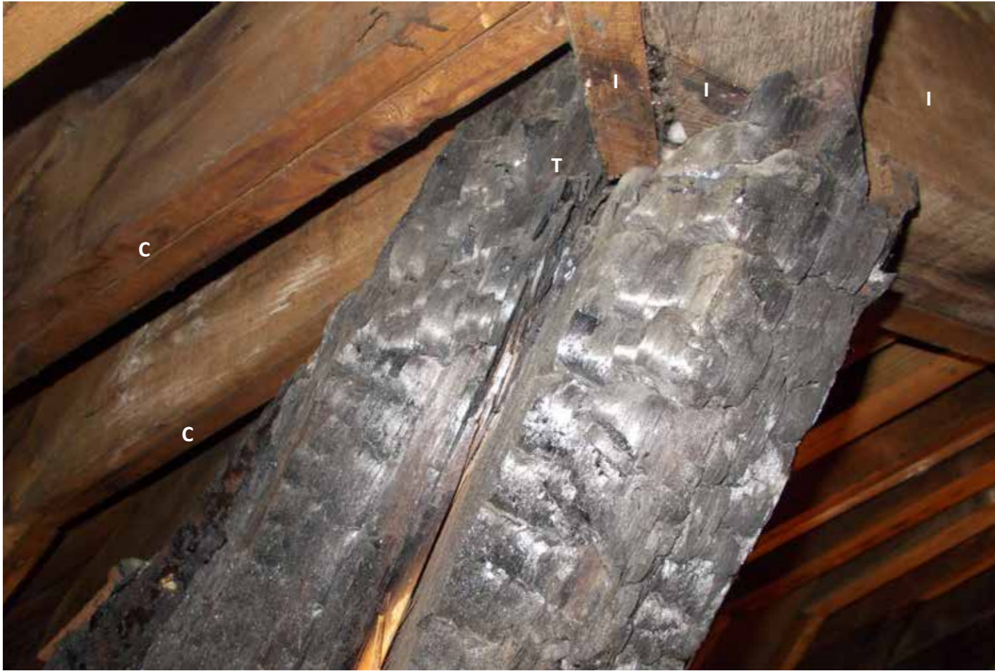
Figure 17: View of junction between the trusses tie beam, 2-part ribs and the inner apex ring beam. Note previous fire damage (possibly in the early 20th C). (2019) © H&R
