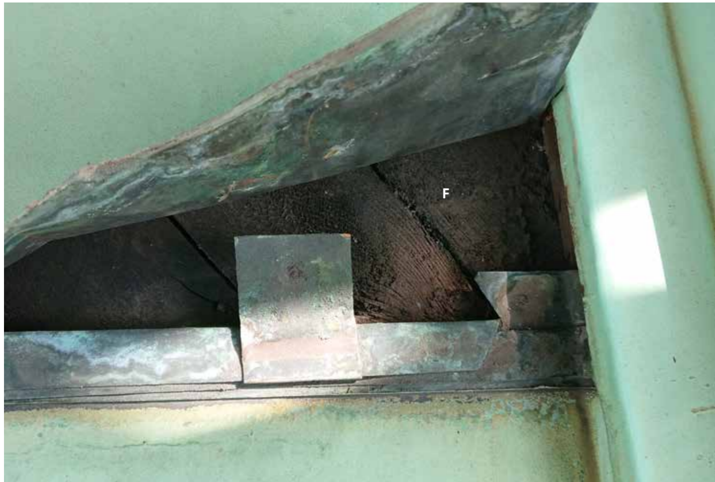
Figure 23: Exterior copper roof cladding and indication of roof boarding beneath the cladding (2019) © H&R
