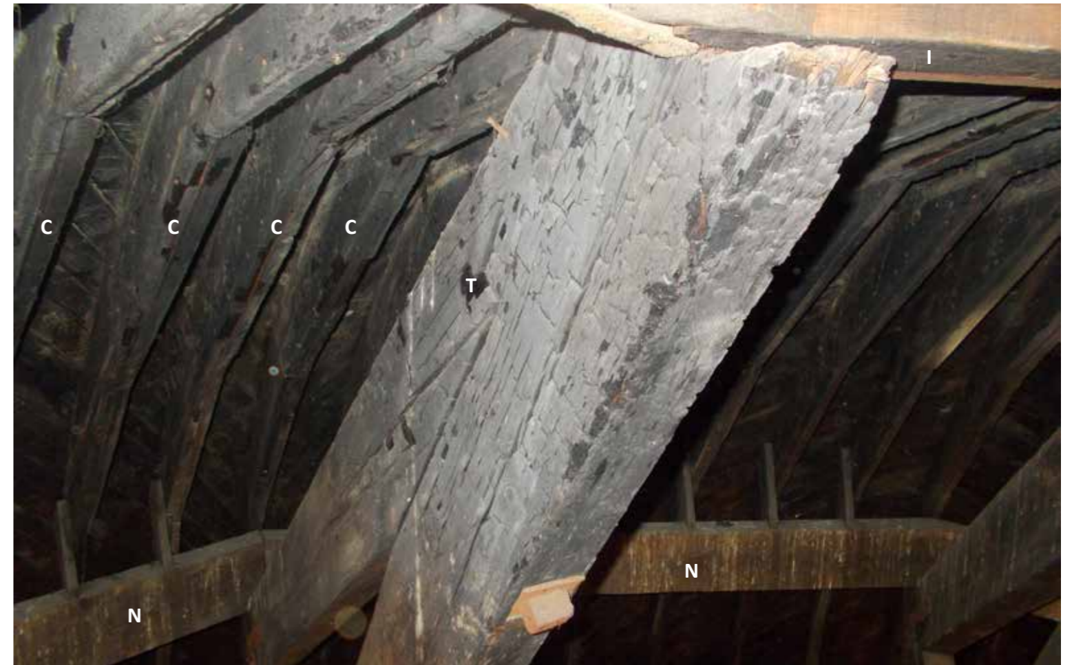
Figure 15: Birds-mouth joint between the truss and inner apex ring beam. Note previous fire damage (possibly in the early 20th C). (2019) © H&R
