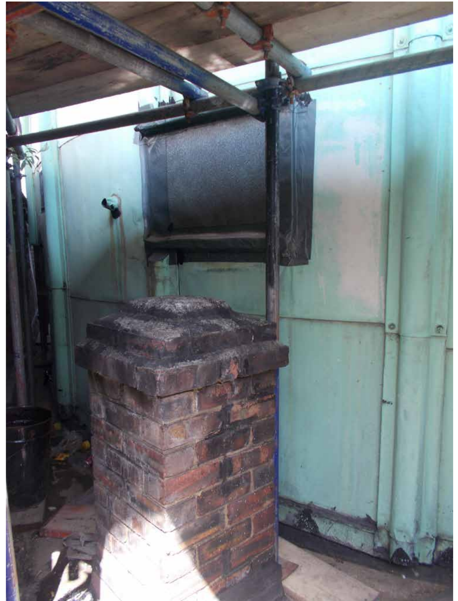
Figure 25: Exterior view of dome wall, next to brick pier on NW side of the building (2019) © H&R
