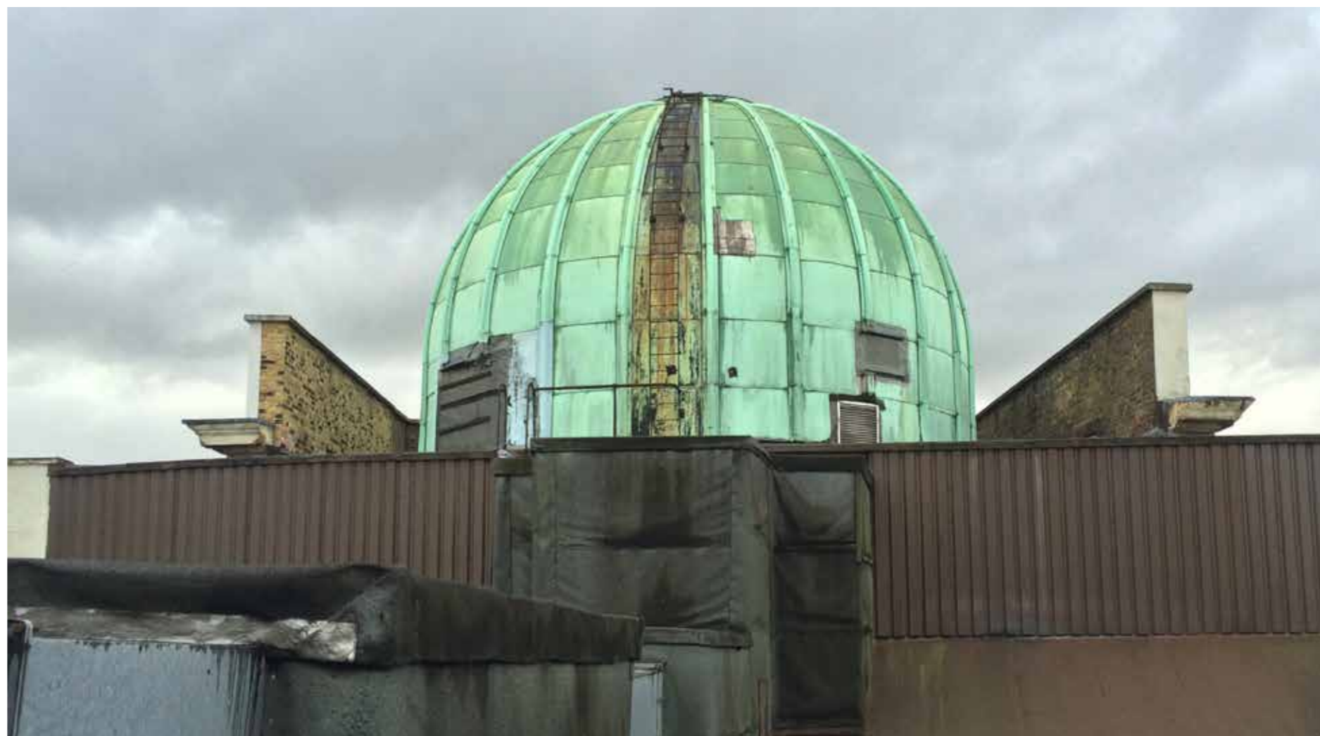
Figure 2: KOKO Dome condition pre-fire (2018). © SLHA
