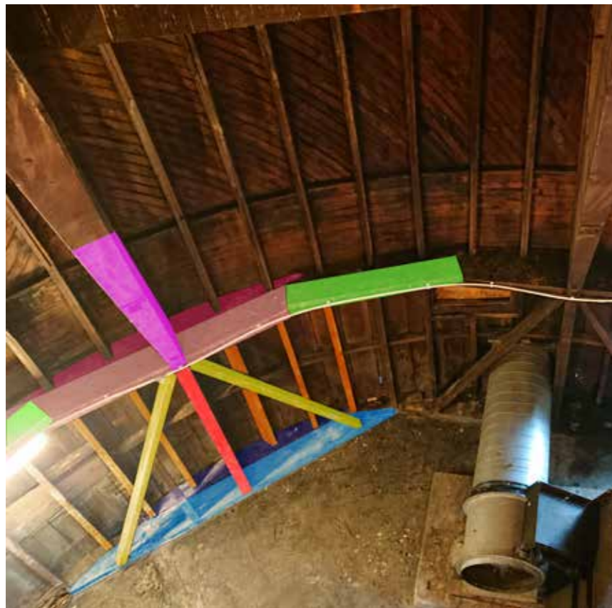
Figure 39: Various principle elements (Main support post with braces, upper rafter plate, lower stud wall plate), king post truss and horizontal rafter wall ties) indicated in situ (2019) © H&R (SLHA edit)
