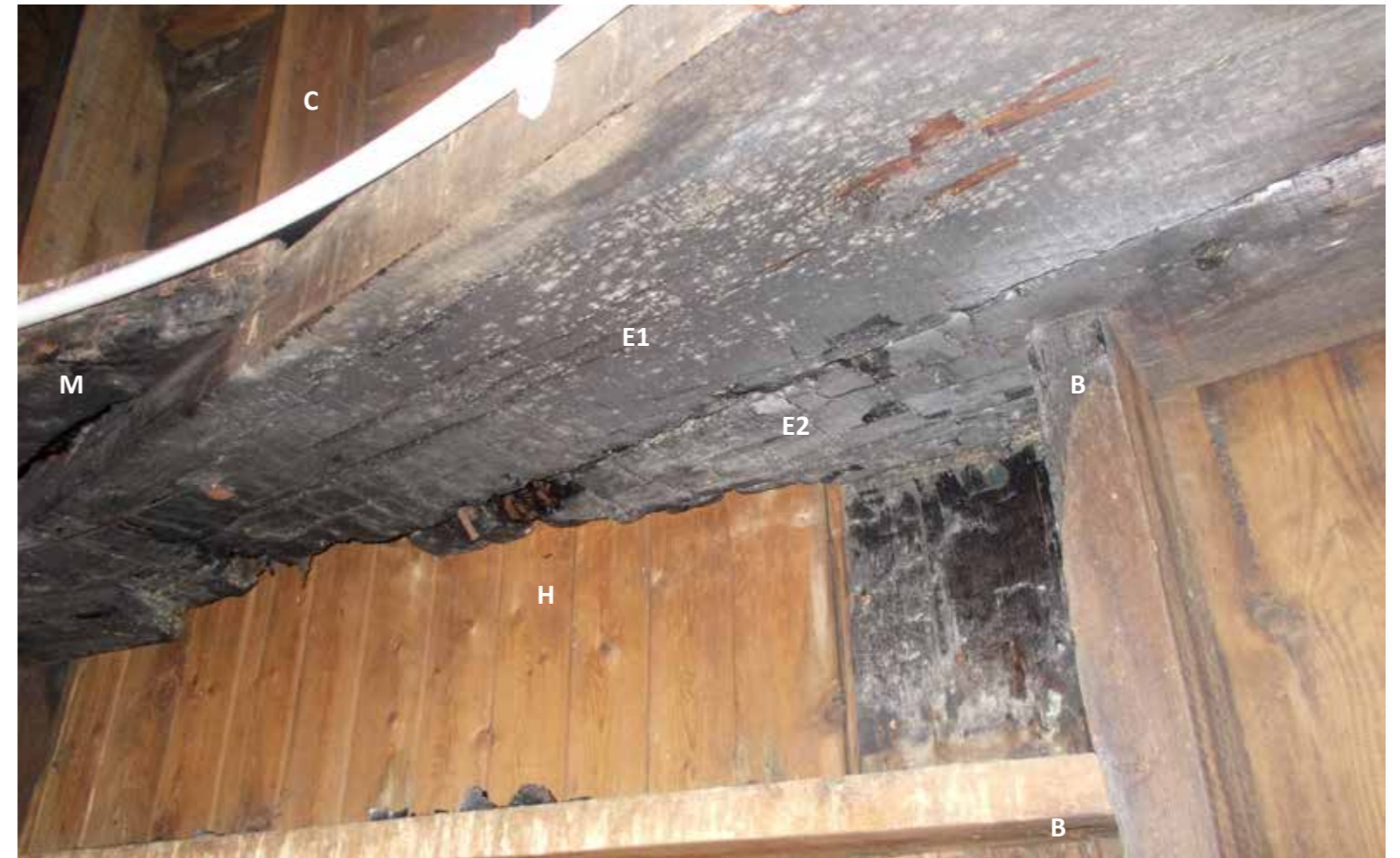
Figure 21: Bottom view of upper rafter plate. Note previous fire damage (possibly in the early 20th C). (2019) © H&R
