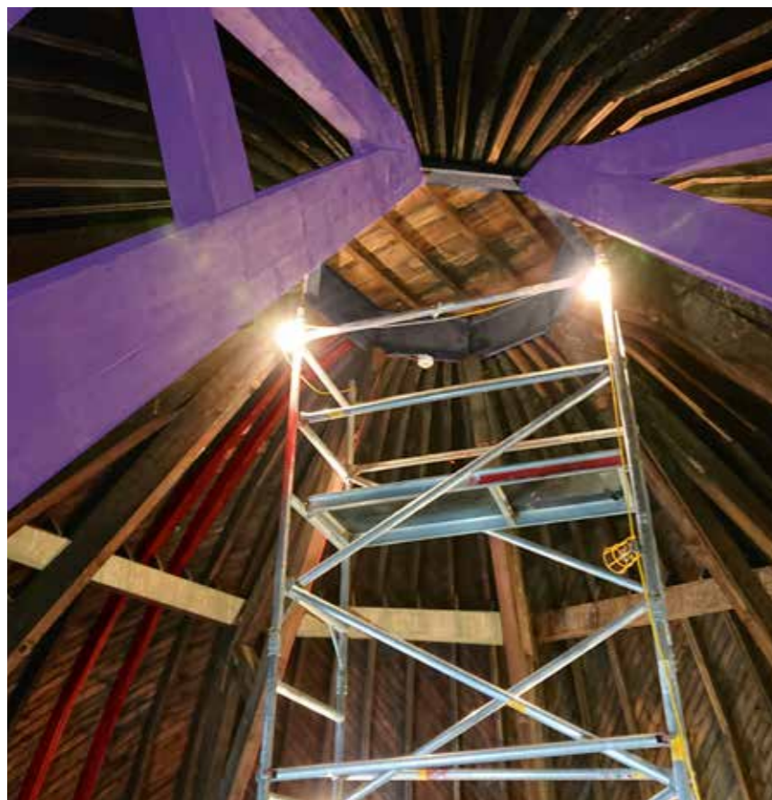
Figure 36: Various principle elements (Inner apex ring beam, King post truss, 2-Part ribs and Truss purlins) indicated in situ (2019) © H&R (SLHA edit)
