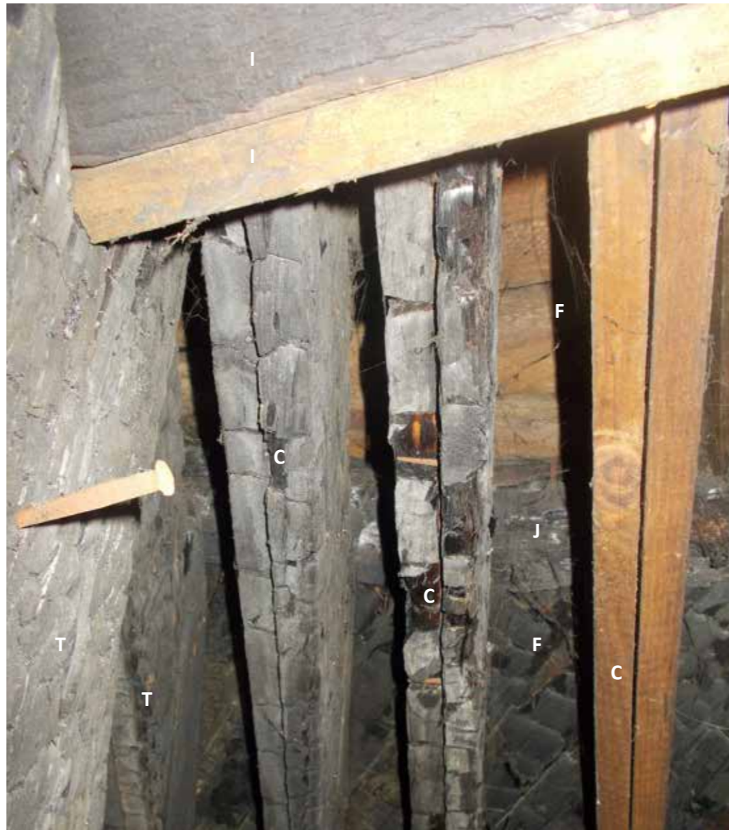
Figure 10: 2-part timber ribs at apex junction & birds-mouth (shown on the left corner) joint from end tie beam of truss. Note previous fire damage (possibly in the early 20th C). (2019) © H&R
