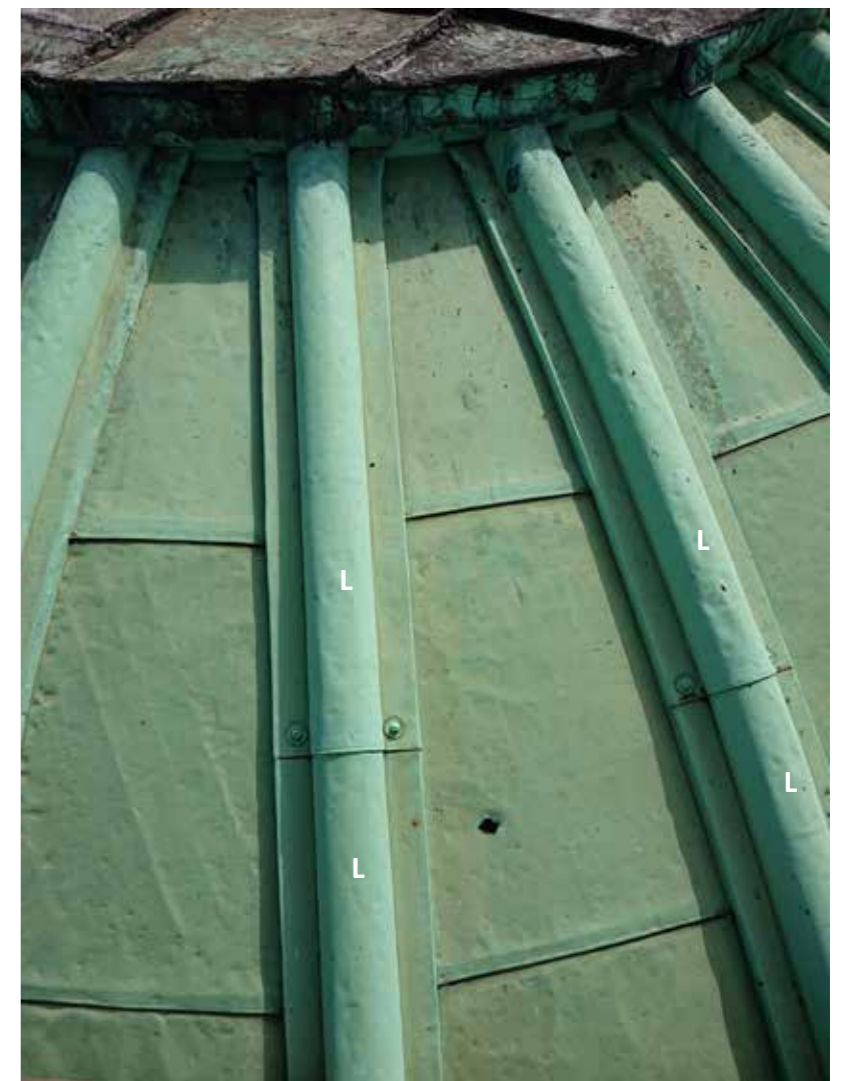
Figure 13: Ribs of dome exterior shaped by timber roof rolls (2019) © H&R (Please note: Annotation (L) is beneath the copper roof sheet)
