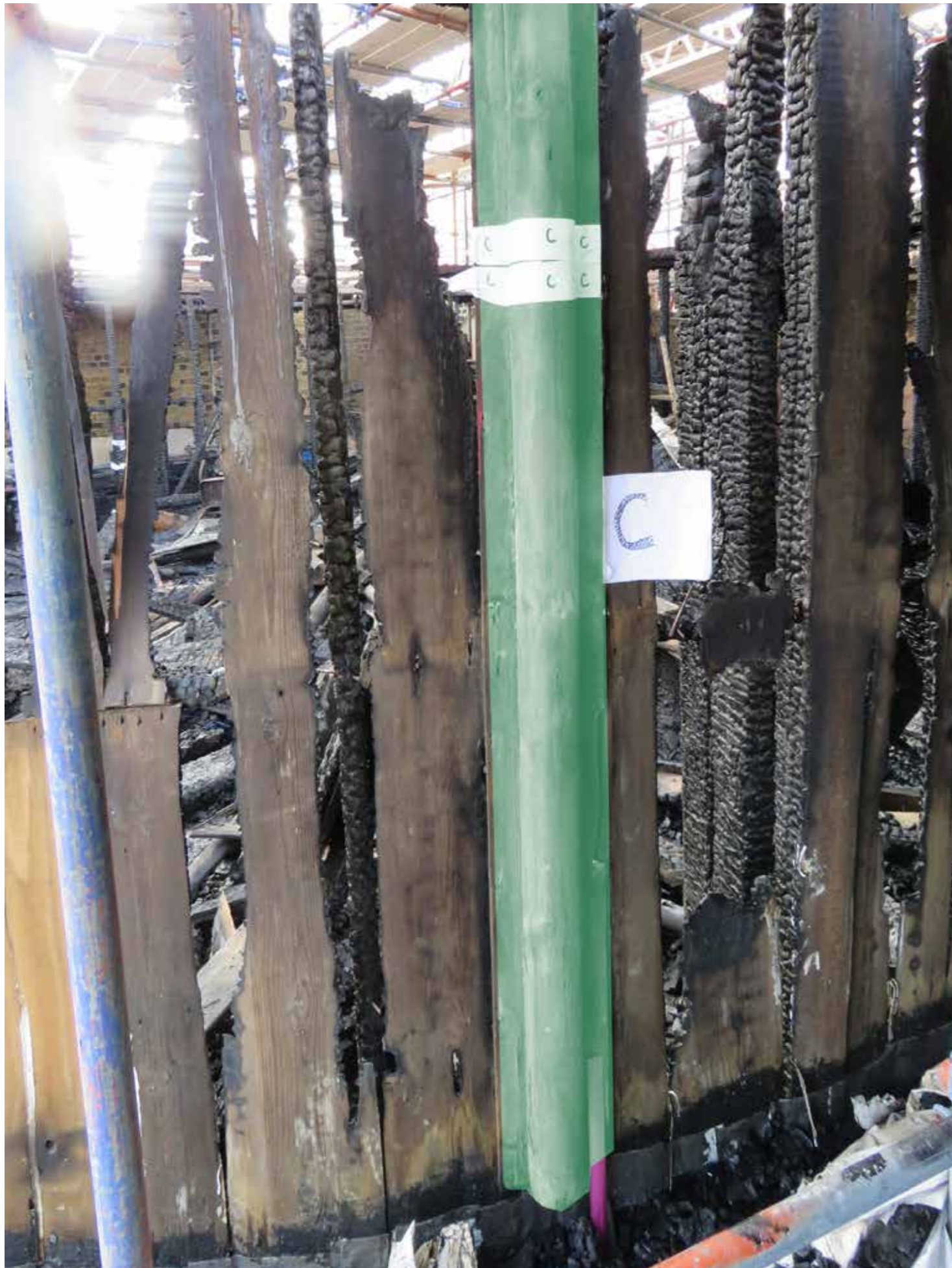
Figure 125: Sample #18- Timber roof rolls (L) at base level with wall boarding (H) in situ (incorrect label during site survey) (2020) © SLHA
