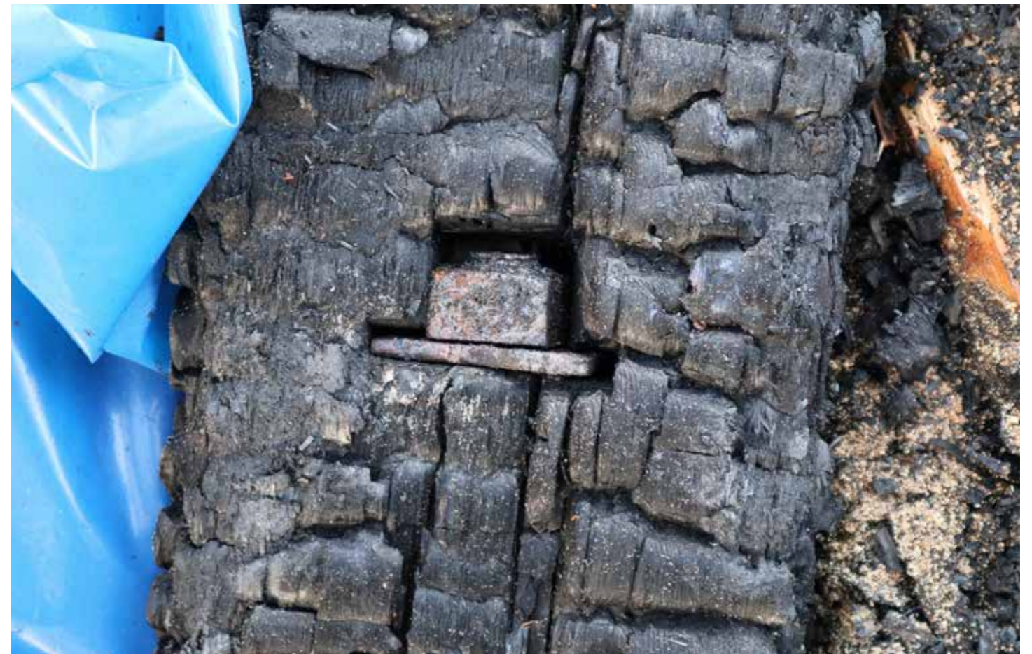
Figure 156: Bolted metal brace (T4) connecting king post (T2) to tie beam (T1) in situ (2020) © SLHA
