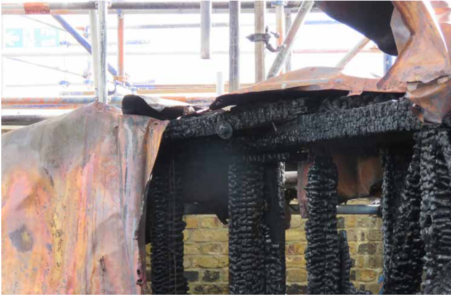
Figure 145: Horizontal rafter wall ties (M) with upper rafter plate (E) in situ (2020) © SLHA
