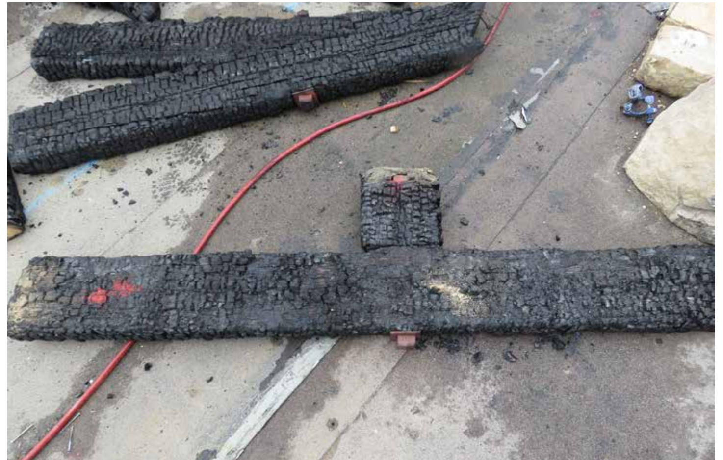
Figure 160: Sample #26 - Bolted metal brace (T4) connecting king post (T2) to tie beam (T1) in situ (2020) © SLHA
