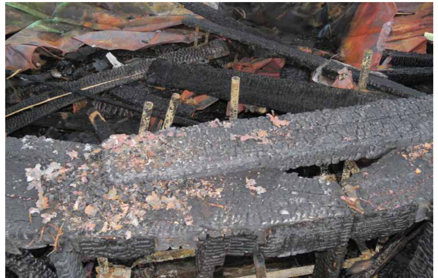
Figure 144: Horizontal rafter wall ties (M) with upper rafter plate (E) in situ (2020) © SLHA
