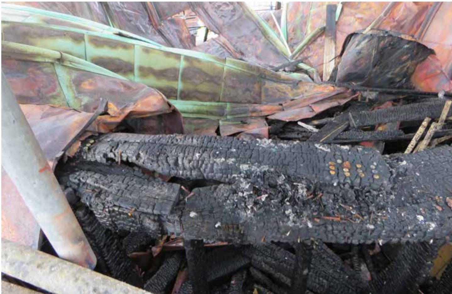
Figure 146: Horizontal rafter wall ties (M) with upper rafter plate (E) in situ (2020) © SLHA
