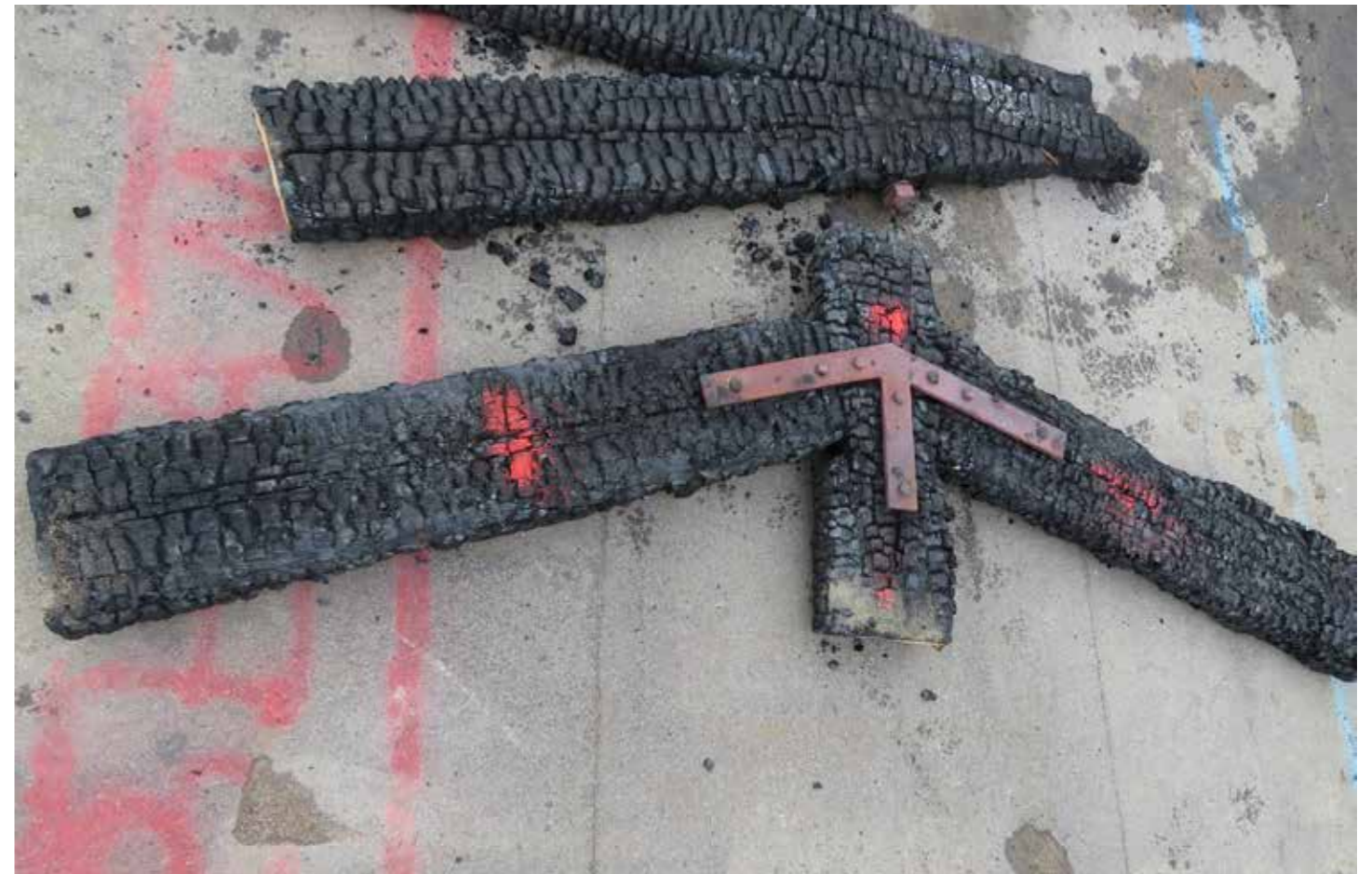
Figure 159: Sample #25 - Bolted arrowhead metal brace (T4) connecting king post (T2) to principal rafters (T3) sample taken (2020) © SLHA
