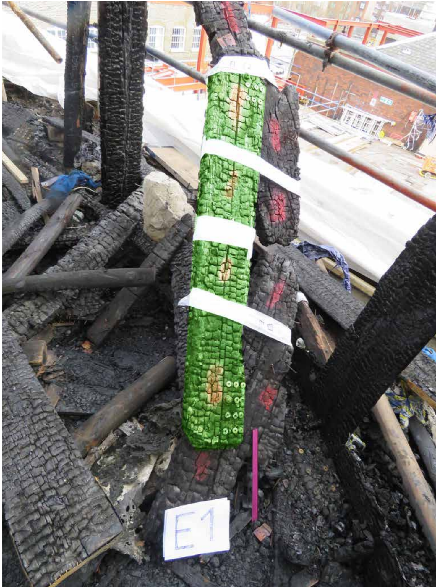
Figure 139: Sample #20 - Horizontal rafter wall ties (M) with upper rafter plate (E) - sample taken (2020) © SLHA
