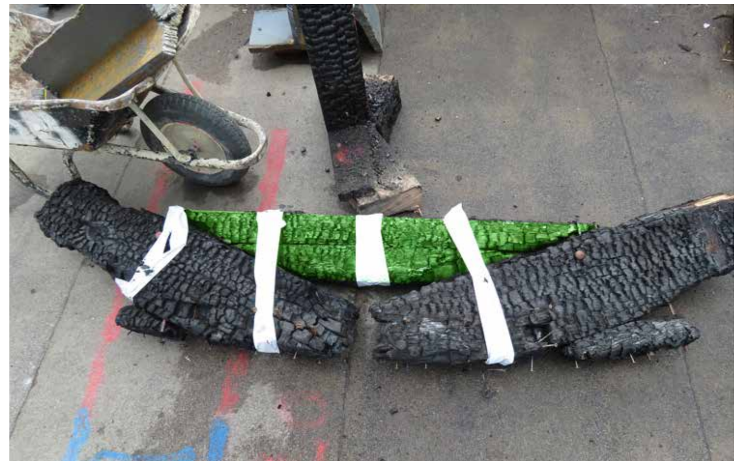
Figure 141: Sample #20 - Horizontal rafter wall ties (M) with upper after plate (E) - sample taken (2020) © SLHA
