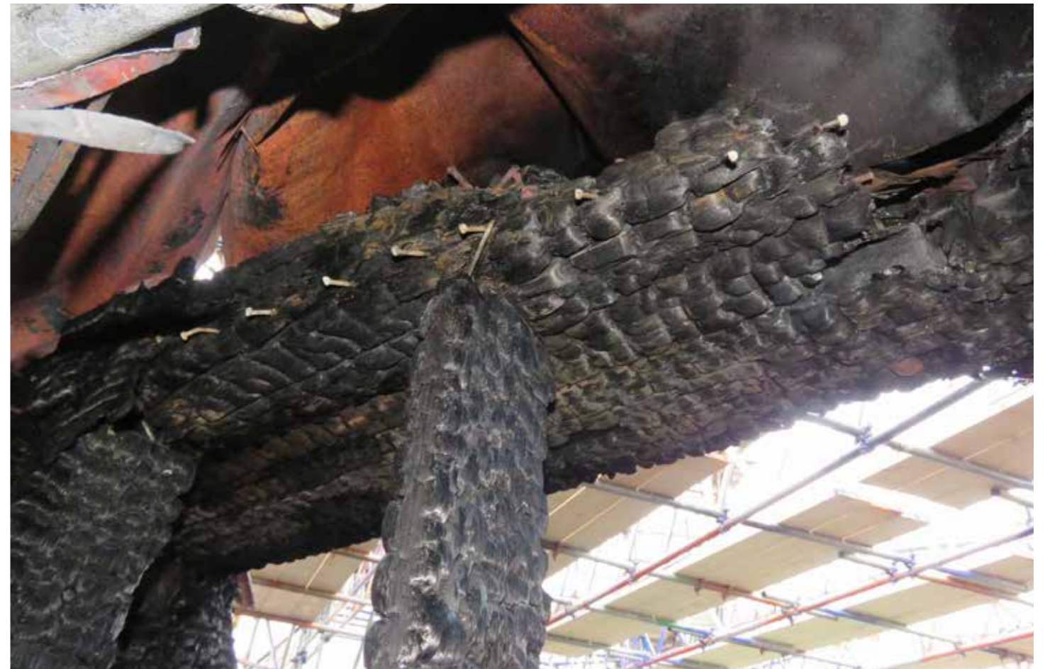
Figure 97: Outer upper rafter plates (E2) with wall stud (B) in situ (2020) © SLHA
