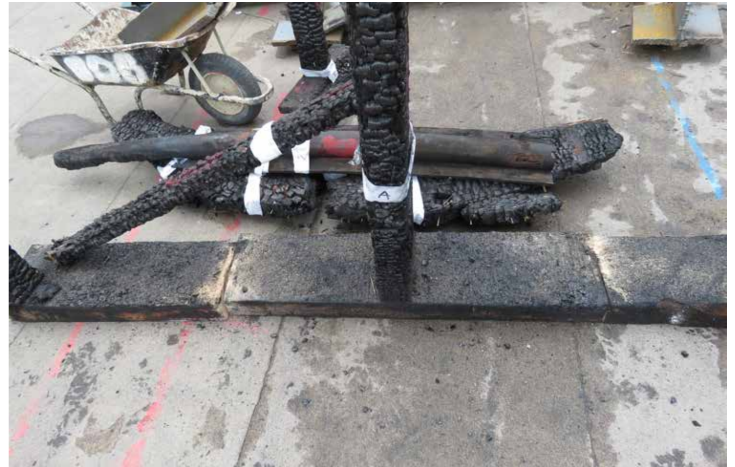
Figure 83: Sample #13 - Inner lower stud wall plate (D1) with main support post (A) and supporting braces (G). This elements was required to be divided into three separate parts (2020) © SLHA
