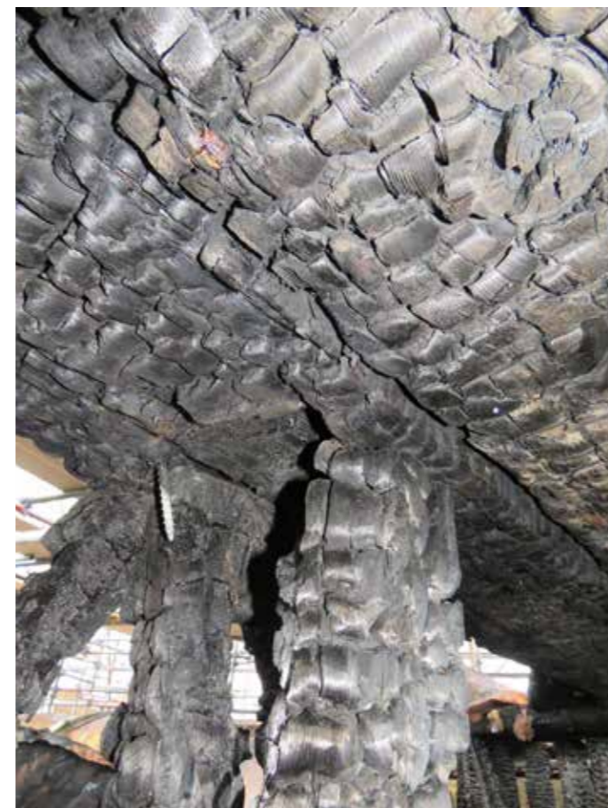
Figure 98: Upper rafter plates (E) with wall stud (B), main support post (A) and braces (G) in situ (2020) © SLHA
