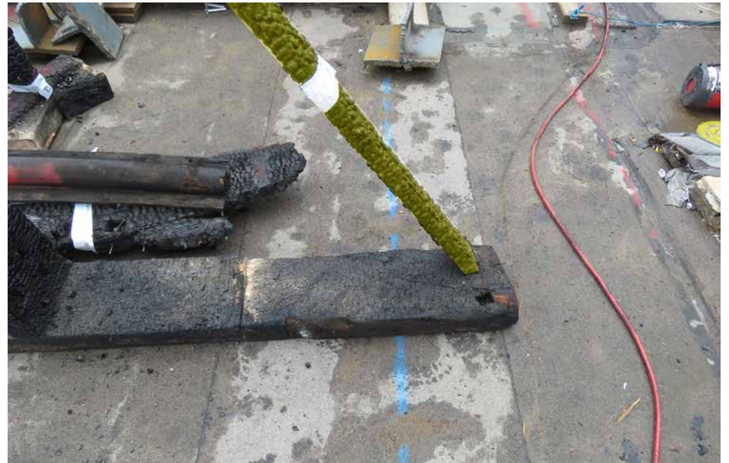
Figure 45: Sample #1 - Main support posts braces (G) on inner lower stud wall (D) (2020) © SLHA
