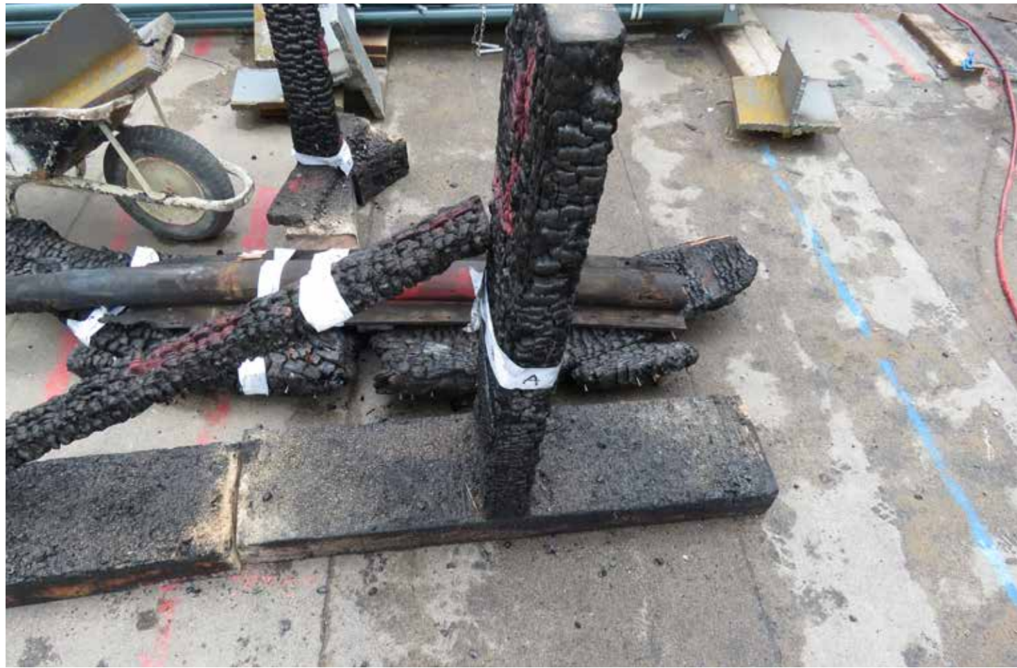
Figure 50: Sample #3 - Main support posts (A) and lower stud wall plate (D) (2020) © SLHA
