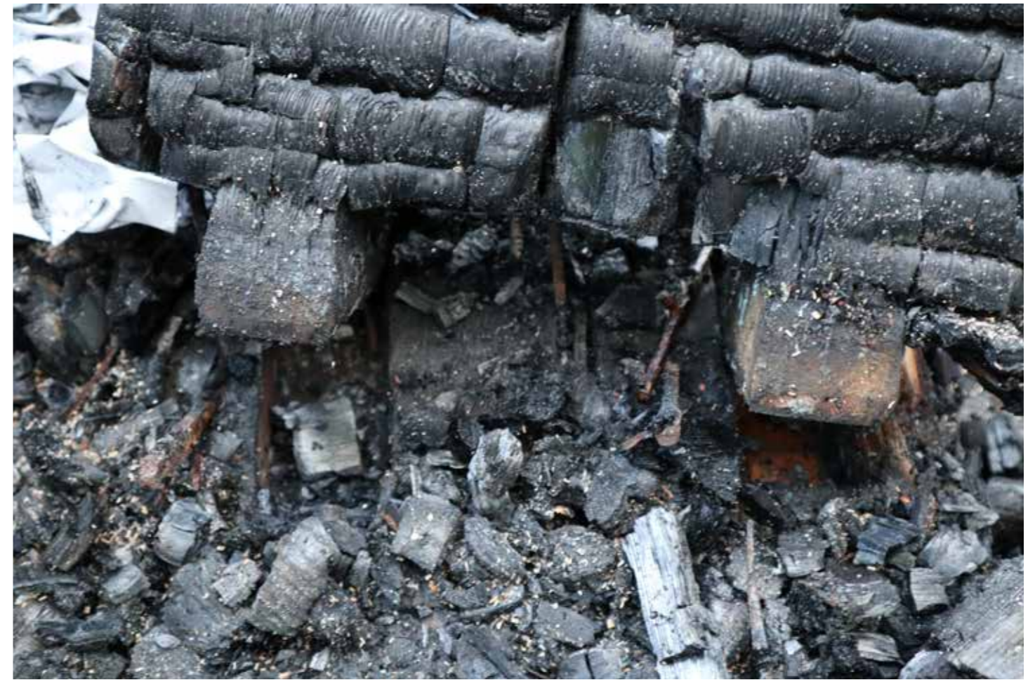
Figure 48: Mortise and tenon joints between main support posts (A) and lower stud wall plate (D) (2020) © SLHA
