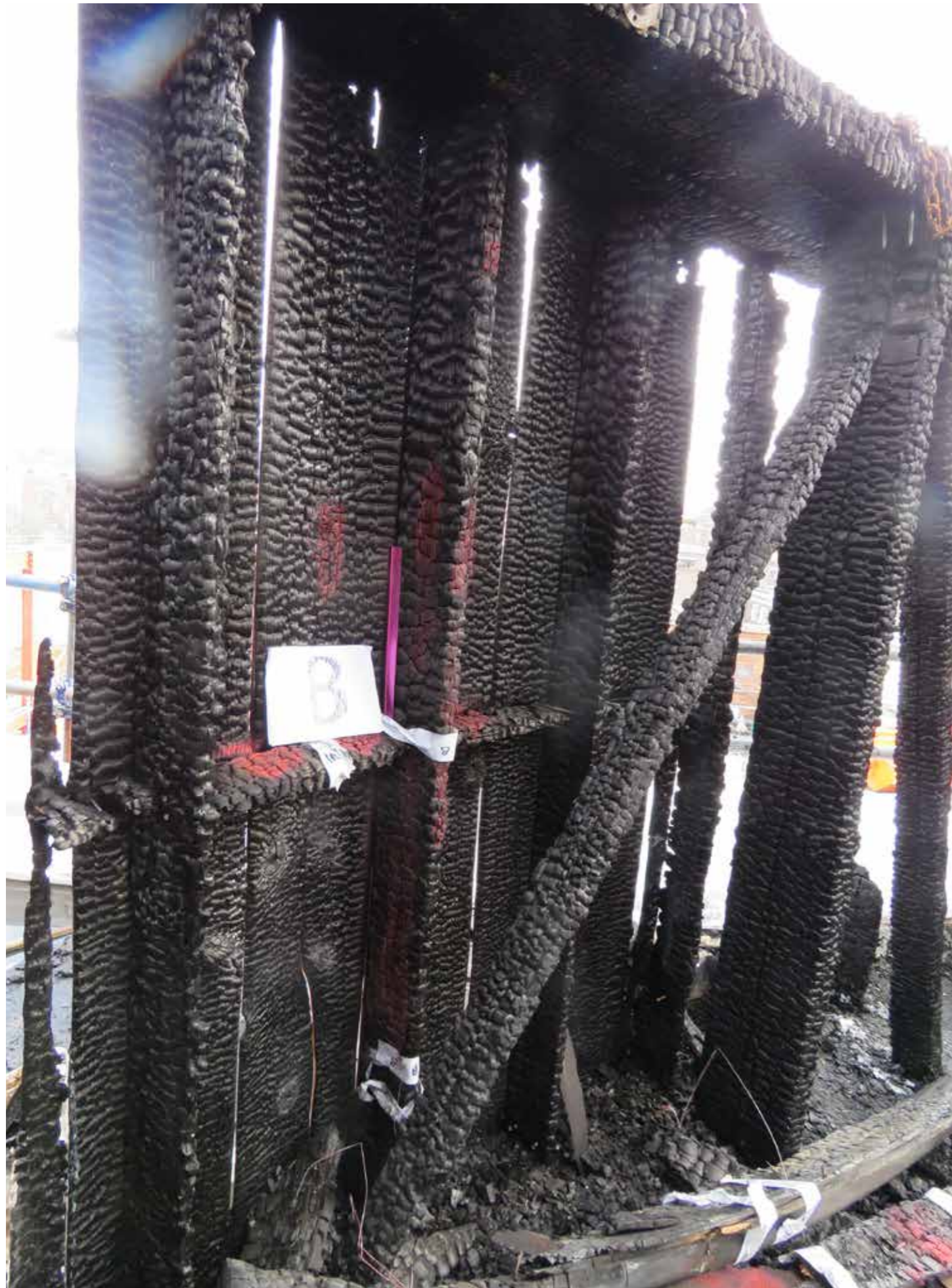
Figure 61: Wall studs and ties (B) in situ with wall boarding (H) and indication of proximity to main support posts (A) (2020) © SLHA
