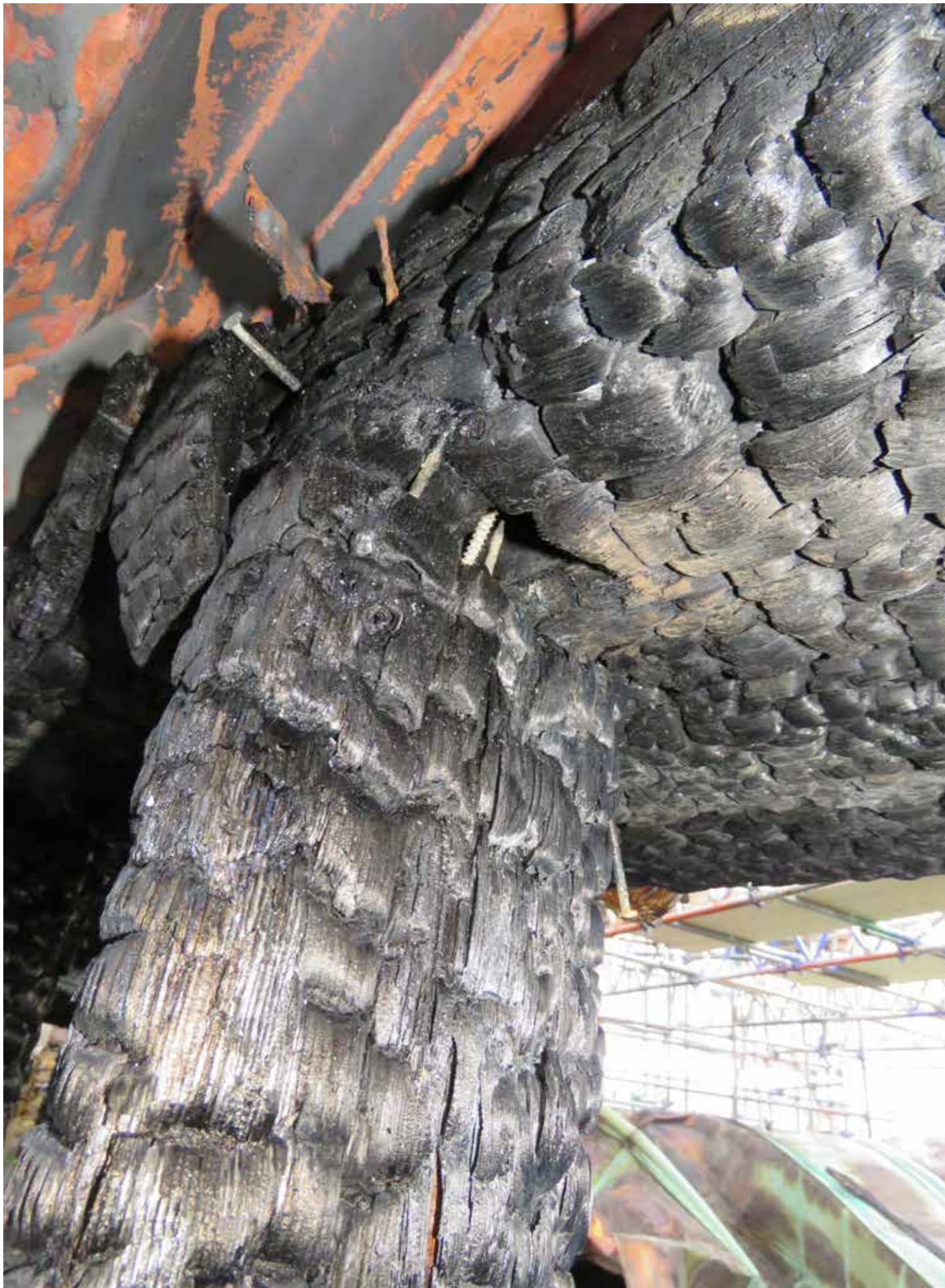
Figure 96: Outer upper rafter plates (E2) with wall stud (B) in situ (2020) © SLHA
