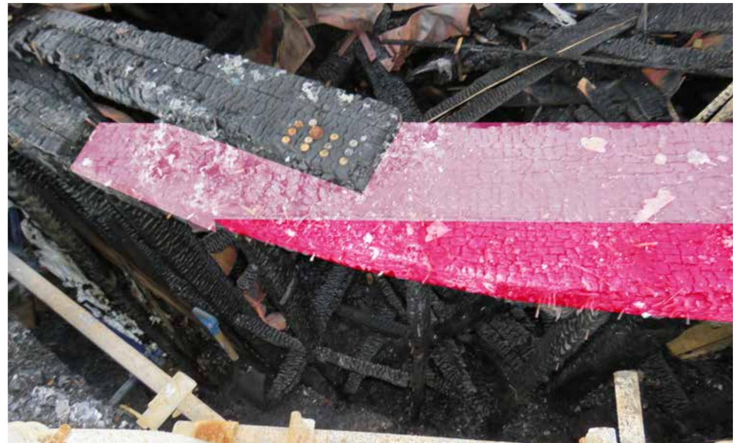
Figure 95: Upper rafter plates (E) with corresponding horizontal rafter wall tie (M) in situ (2020) © SLHA
