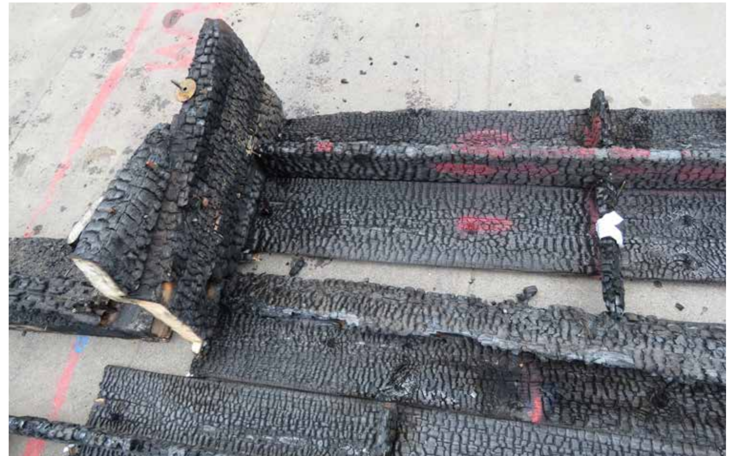
Figure 67: Sample #6 - Wall stud (B) with upper rafter plate (D), wall boarding (H) and horizontal rafter wall tie (M) (2020) © SLHA
