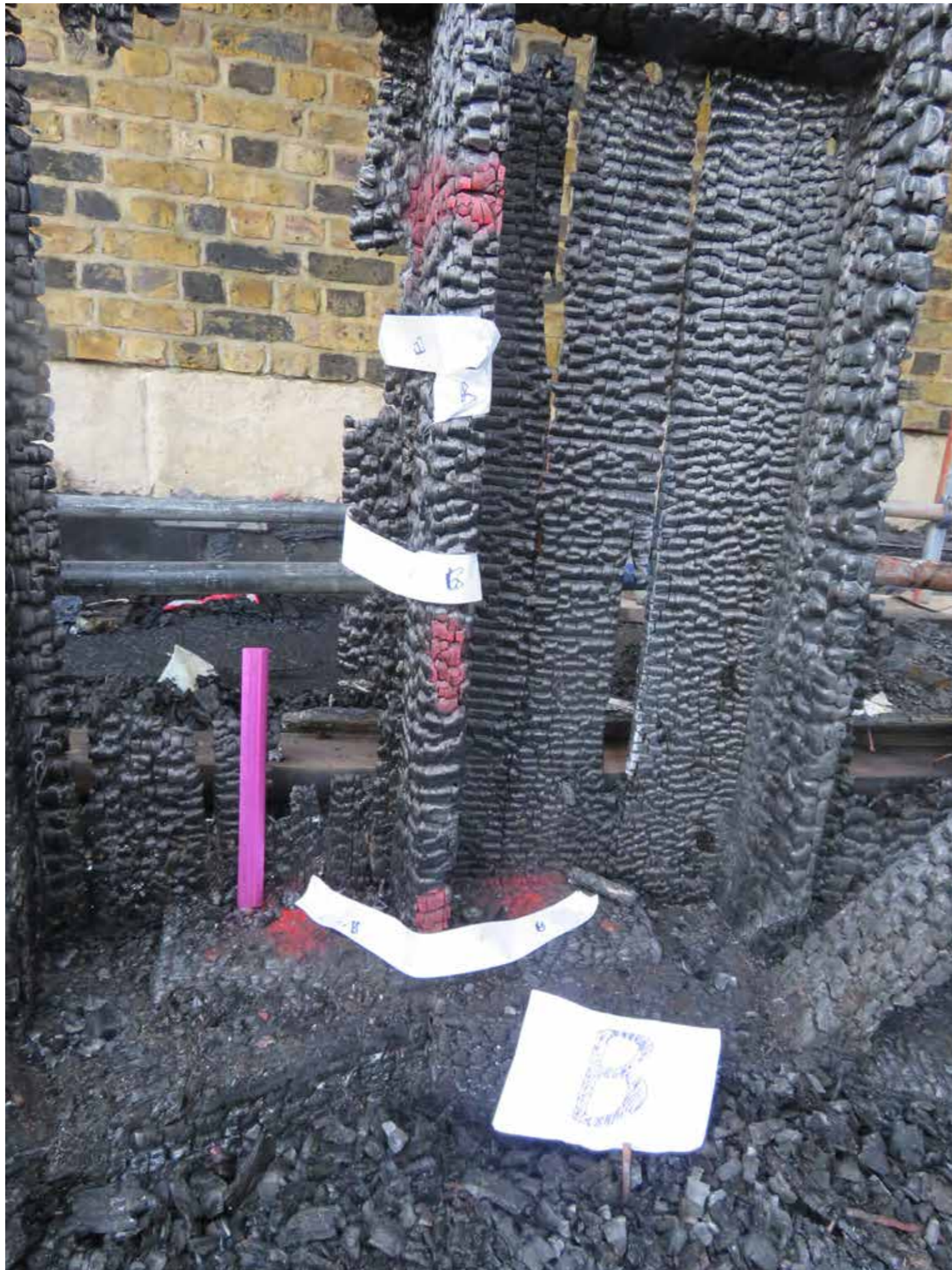
Figure 65: Wall studs (B) with bottom plate connecting the lower stud walls (D) in situ (2020) © SLHA
