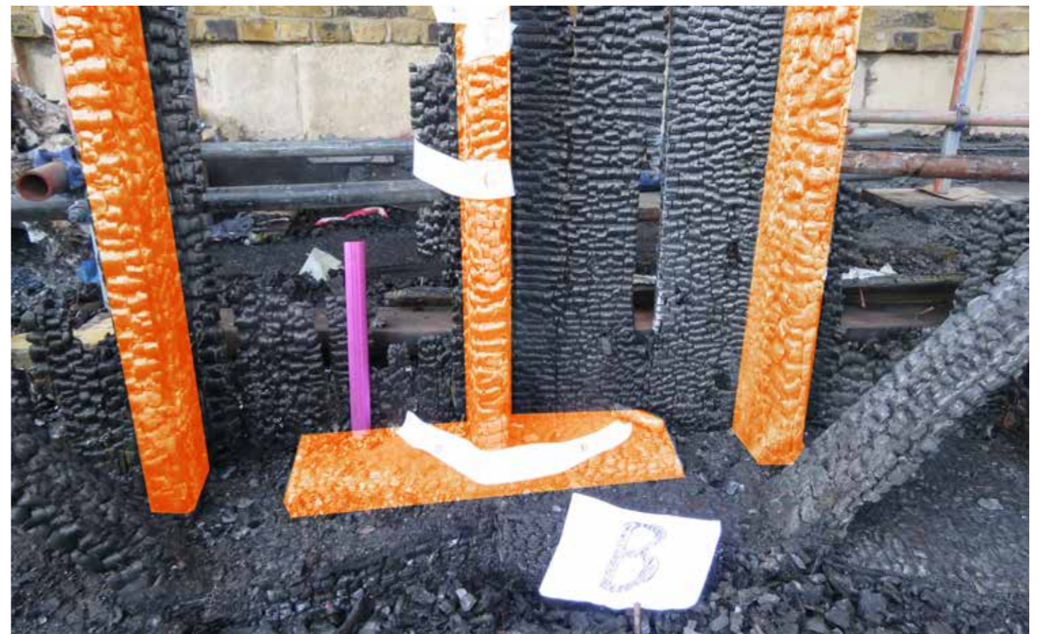
Figure 60: Wall studs (B) with bottom plate tie at junction between the corner of lower rafter plates (2020) © SLHA
