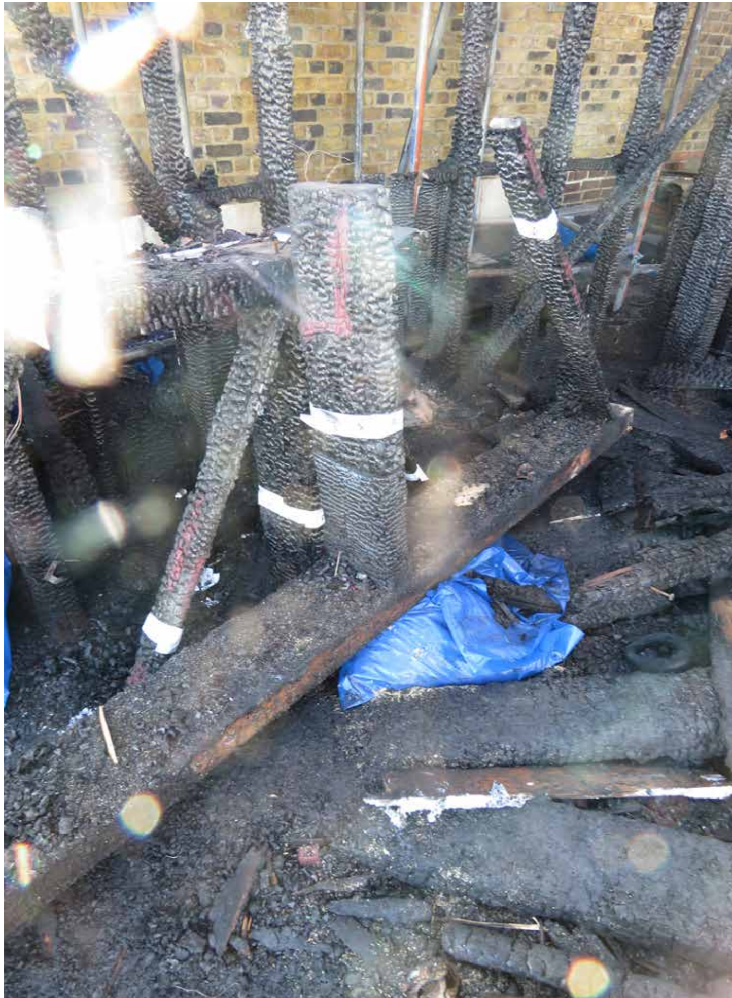
Figure 85: Sample #13 - Inner lower stud wall plate (D1) with main support post (A) and supporting braces (G). (2020) © SLHA
