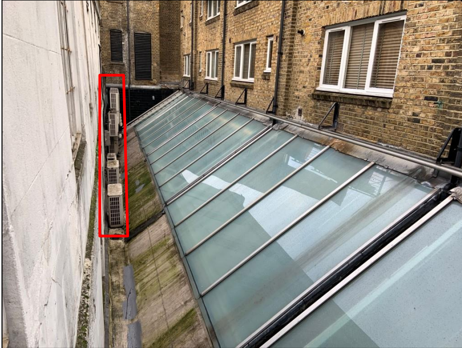
Figure 3 Existing outdoor air-conditioning units located on 24 West Street rear facade to be removed/replaced
