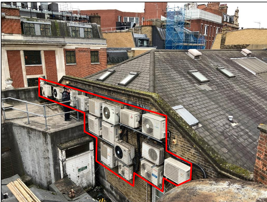
Figure 4 Existing outdoor air-conditioning units located on 24 West Street south gable wall to be removed/replaced
