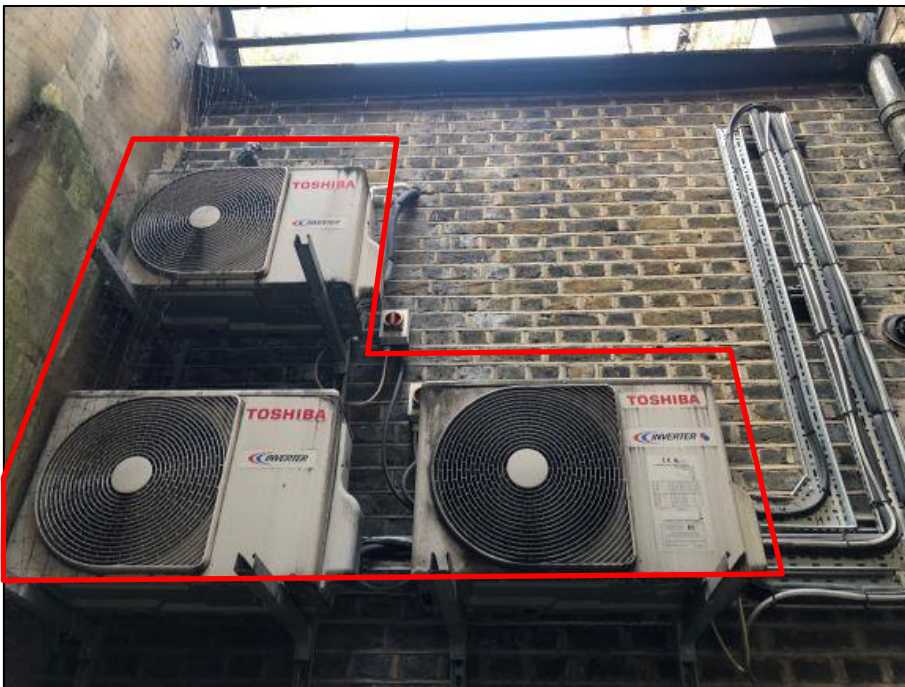
Figure 2 Existing outdoor air-conditioning units located in 26 West Street rear lightwell to be removed/replaced
