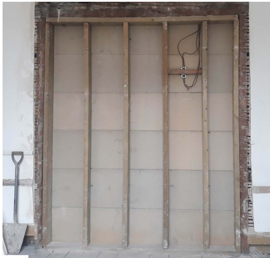
Photograph of existing opening from rear room showing pre-existing timber frame lined with studwork and plasterboard
