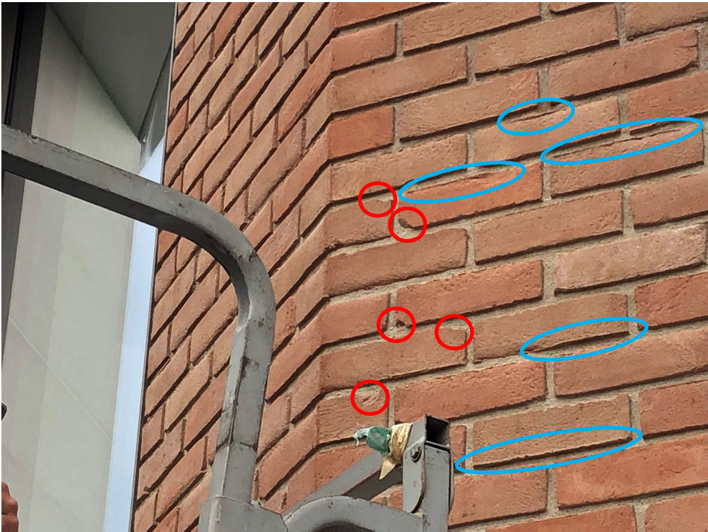
Figure 5 Detail of VMU panel noting lipping to arrises (circled in blue) and dents to corners (circled in red)
