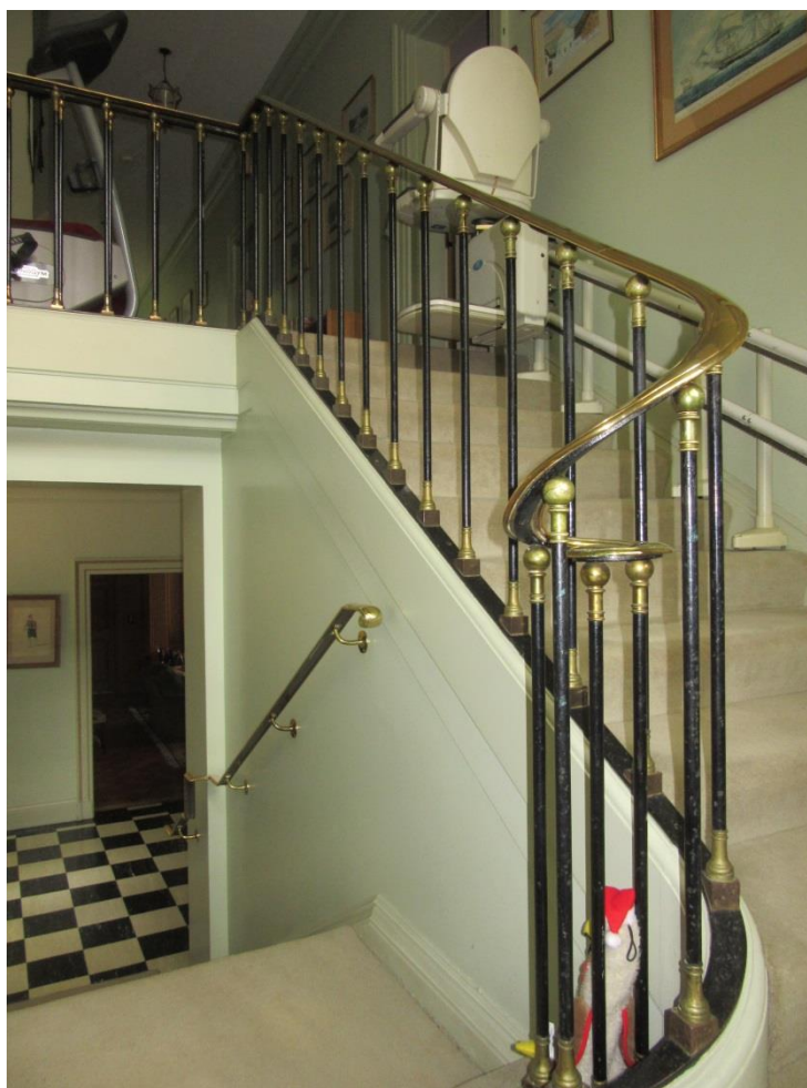
Figure 22: The main staircase with unusual arrangement of balusters and spiral handrail standing commencing at the half landing.
