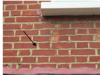
Cracking to front elevation
