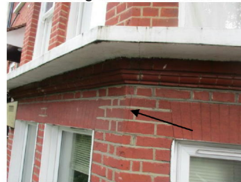
Cracking to right hand bay
