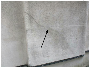
Cracking to right hand flank
