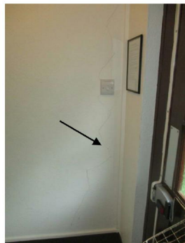
Cracking in communal hall
