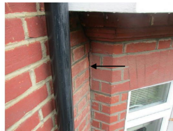
Cracking to right hand bay
