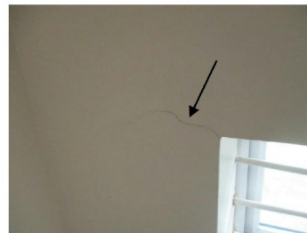
Cracking in communal stairway
