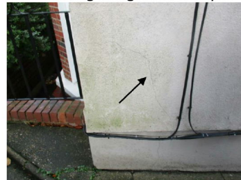
Cracking to right hand flank
