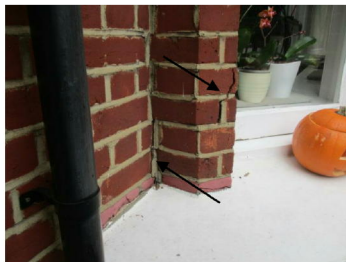
Cracking to right hand bay
