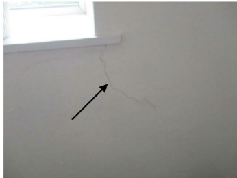
Cracking in communal stairway
