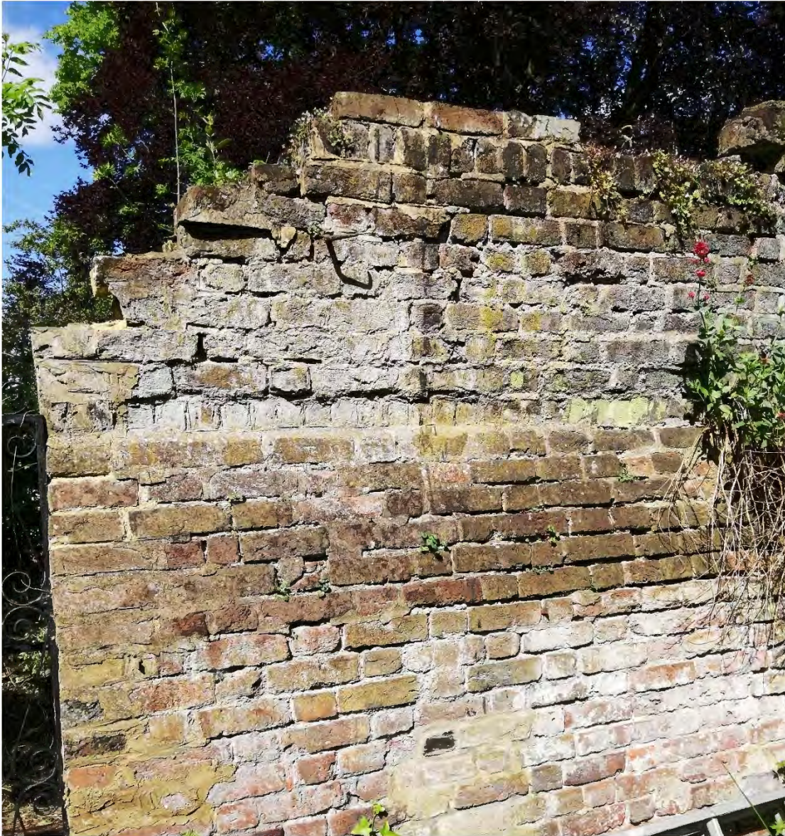
Photo 16, Disrepair at the top of the wall adjacent to Opening 1
