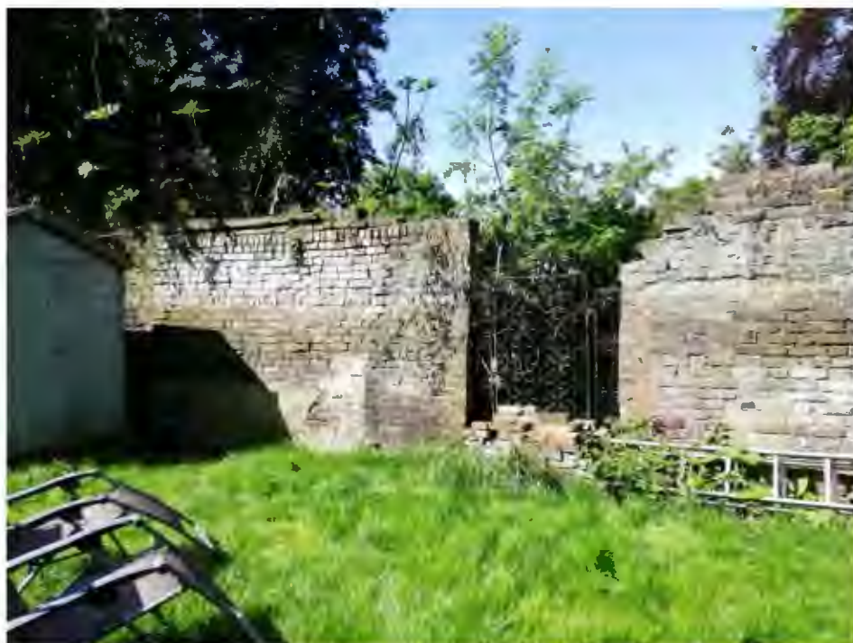
Photo 3, Opening 1, Full height
