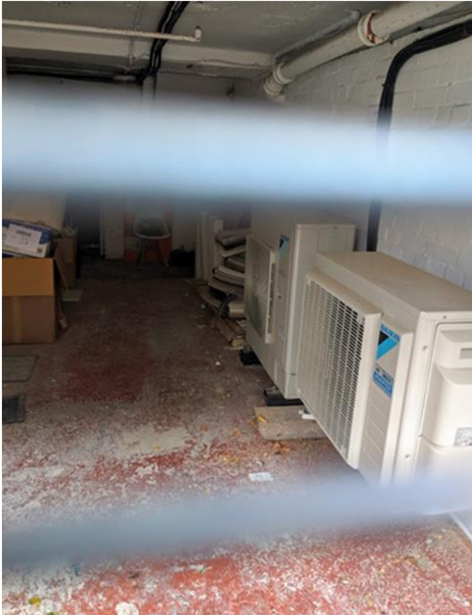
Photo 4: View of lower ground floor garage area including existing air conditioning units
