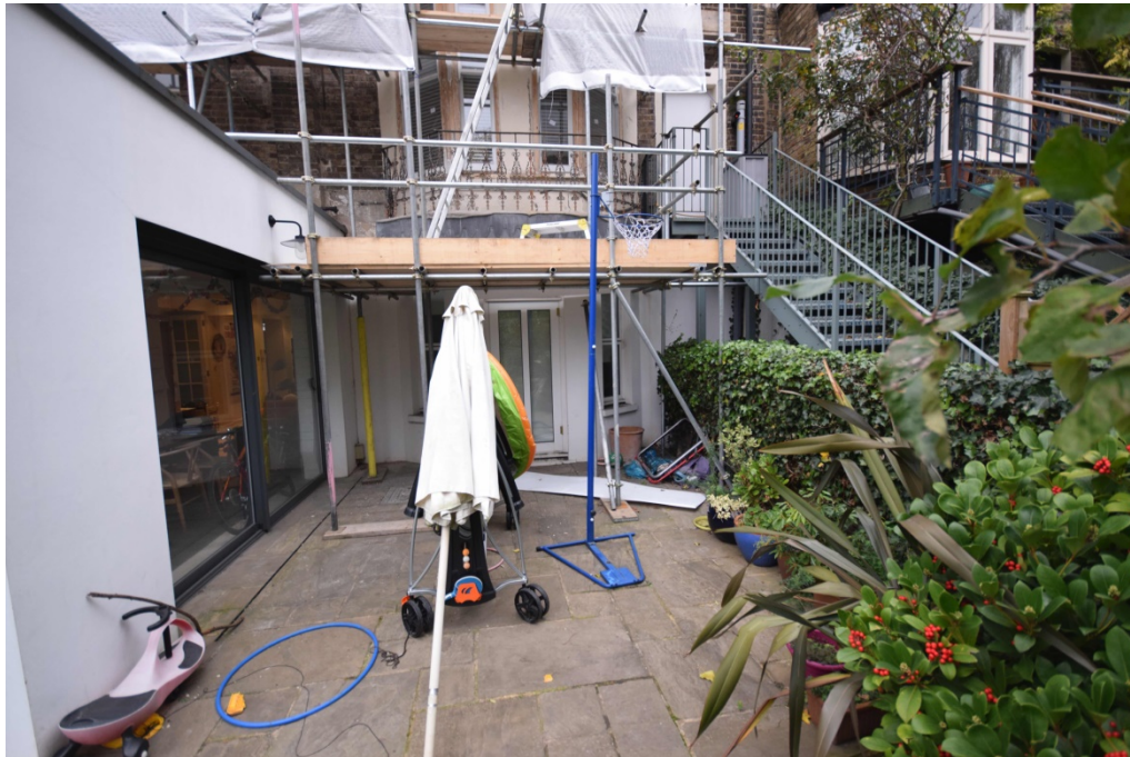
Figure 2: Rear elevation at lower ground floor level showing access stairs to be removed
