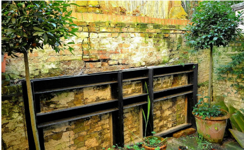
PHOTOGRAPH 03: View showing temporary steel support to damaged lower listed retaining wall as caused by additional loading from raised garden of 31 Willoughby Road.
