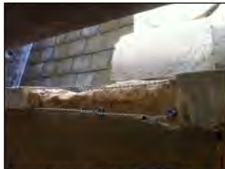
TYPICAL CORNICE REPAIR DETAIL USING HELI BARS AND STAINLESS STEEL TREADED RODS SET IN RESIN
