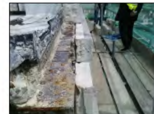
REMOVAL OF STONE PARAPET FOR ACCESS TO CLEAN AND TREAT CORRODING STEEL BEAM
