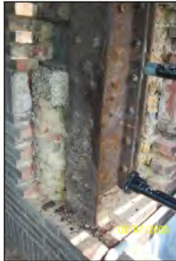
REMOVAL OF BRICKWORK FOR ACCESS TO CLEAN AND TREAT CORRODING STEEL COLUMN
