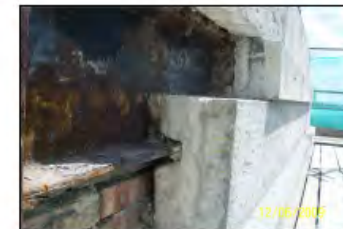
REMOVAL OF STONE PARAPET FOR ACCESS TO CLEAN AND TREAT CORRODING STEEL BEAM
