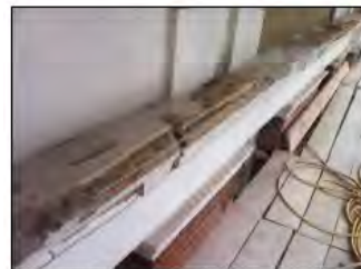
TYPICAL CORNICE REPAIR DETAIL USING HELI BARS AND STAINLESS STEEL TREADED RODS SET IN RESIN
