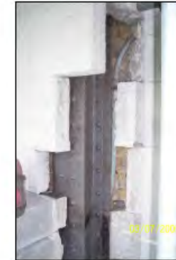
REMOVAL OF STONE FOR ACCESS TO CLEAN AND TREAT CORRODING STEEL COLUMN
