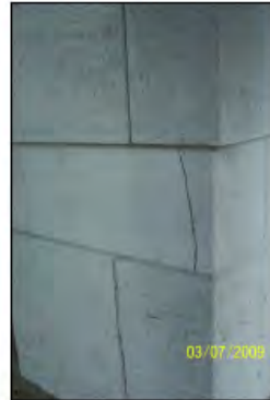
CRACKED STONE CAUSED BY CORROSION OF BURIED STEEL COLUMN BEHIND
