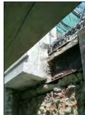
REMOVAL OF STONE PARAPET FOR ACCESS TO CLEAN AND TREAT CORRODING STEEL BEAM
