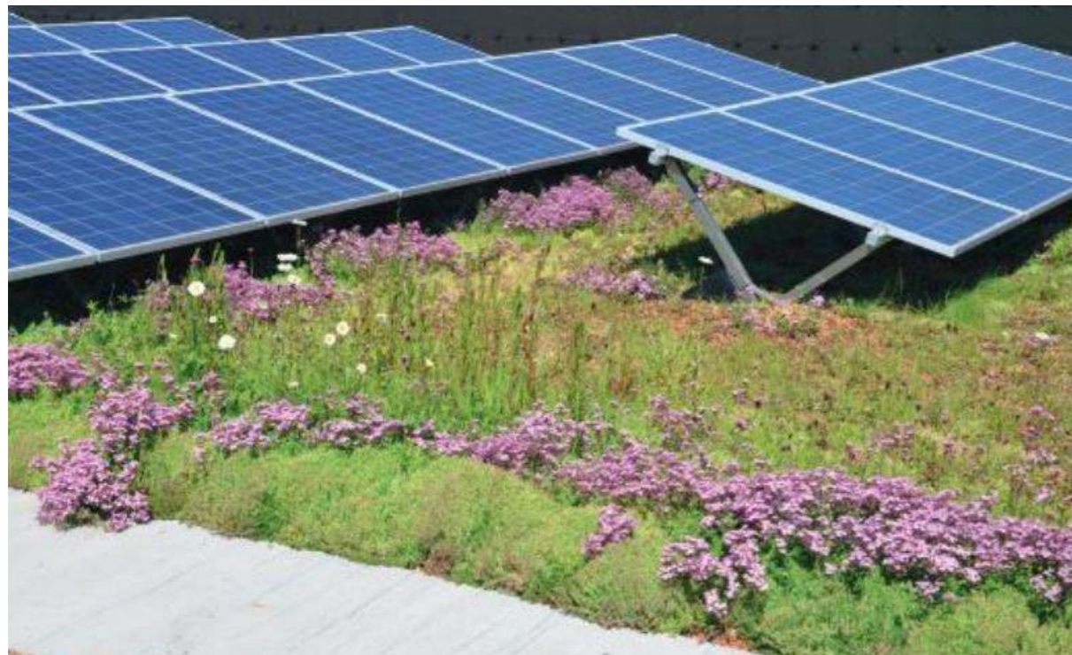
Figure 10 Solar Panel above Green Roof. (Bauder Bisolar)
