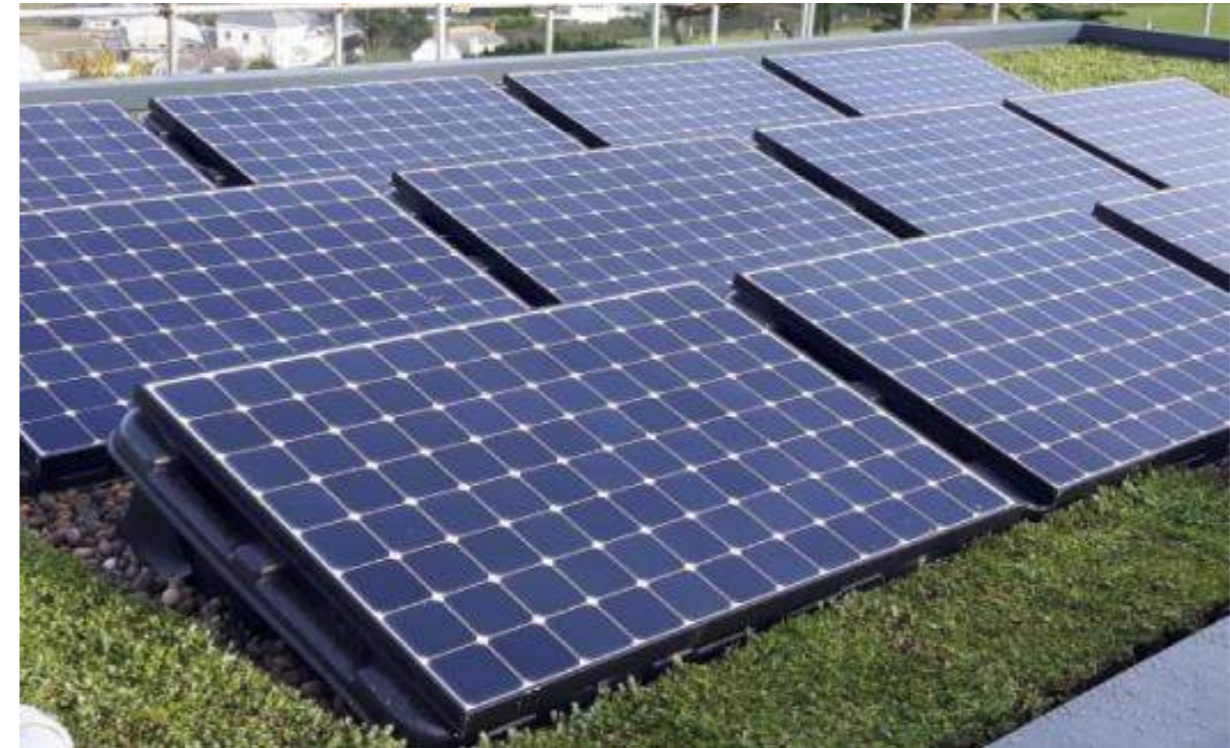
Figure 11 Low Level Solar panel in Green Roof. (Naked Solar)
