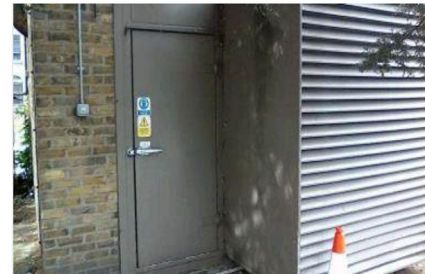
Photo 15. Generator room in the Mortuary building (B5).
