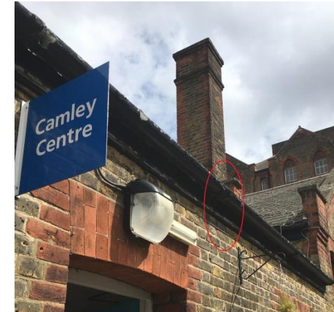
Photo 6. Gap in fascia at Camley Centre (B2).
