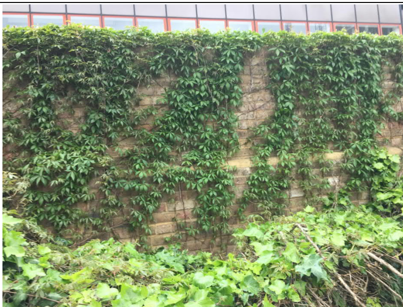
Photo 20. Virginia creeper on the northern boundary of the site.
