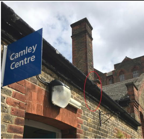
Photo 6. Gap in fascia at Camley Centre (B2).
