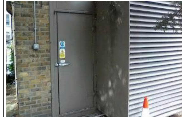
Photo 15. Generator room in the Mortuary building (B5).
