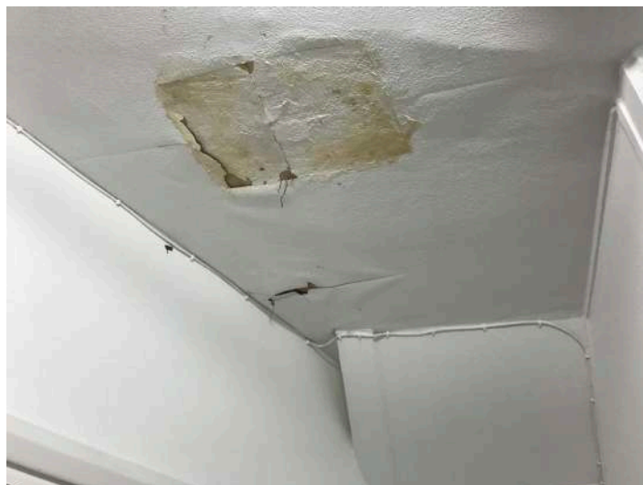
Ceiling showing signs of dump
