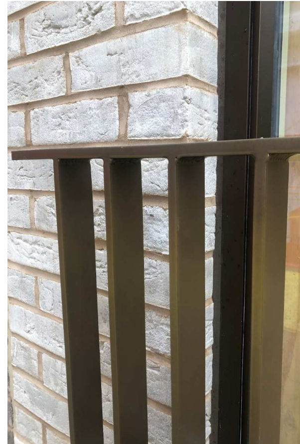
Railing - PPC (Interpon Y2217F Steel Bronze 2) courtyard brick / bronze anodised window frame
