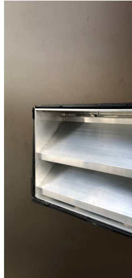
Close-up (incorrect finish)
