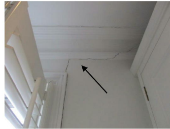
Cracking in 2nd floor front bedroom
