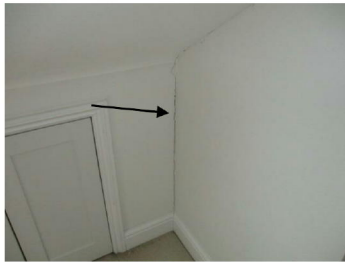
Cracking in loft bedroom
