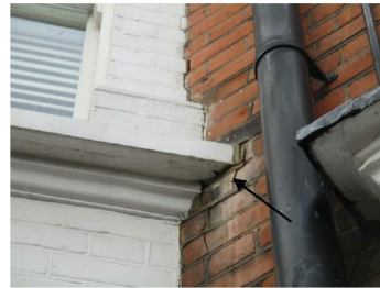
Cracking to front bay
