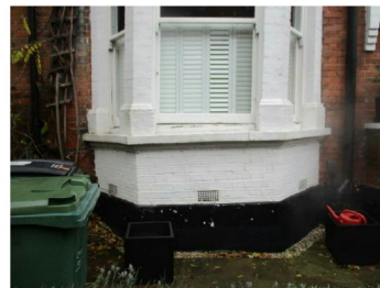
View of historic distortion to front bay
