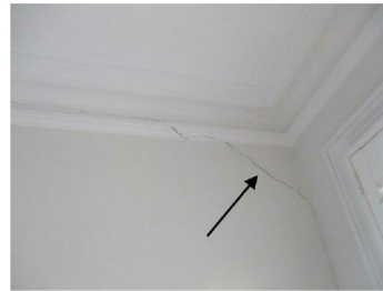
Cracking in 2nd floor front bedroom
