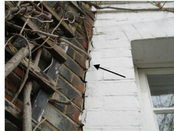
Cracking to front bay
