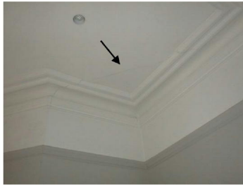
Cracking in lounge
