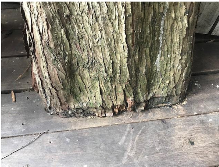
T4- Showing decking damage
