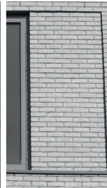
⑤ Example of brickwork reveal detail to front facade alongside windows to study and en-suite
