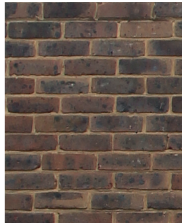
Existing red/ brown brickwork to be cleaned and matched with new brickwork ②
