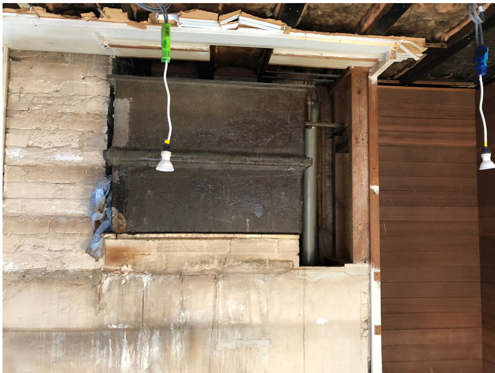
Below: existing leaking water tank causing water damage to wall to be removed
