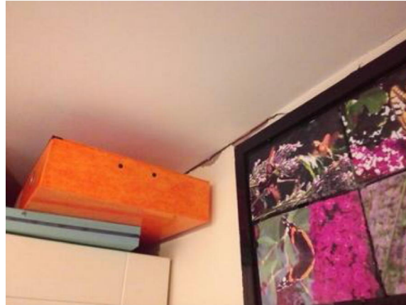
FIGURE 04 Shows cracking inside the office at first floor level of the extension
