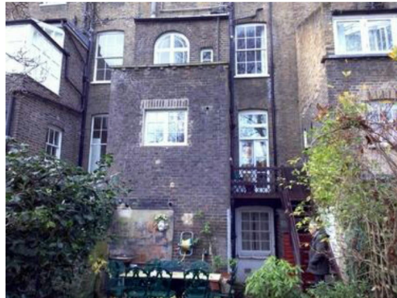
FIGURE 06 Shows the rear elevation of the affected two storey rear extension
