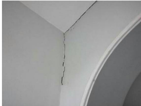
FIGURE 05 Shows cracking inside the upper landing recess which leads onto the roof terrace to rear extension
