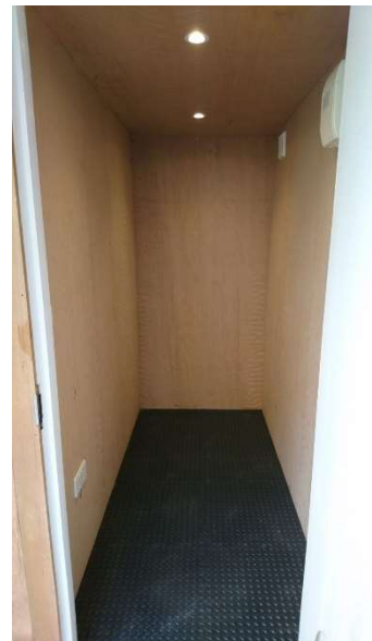
Example of a storage room
