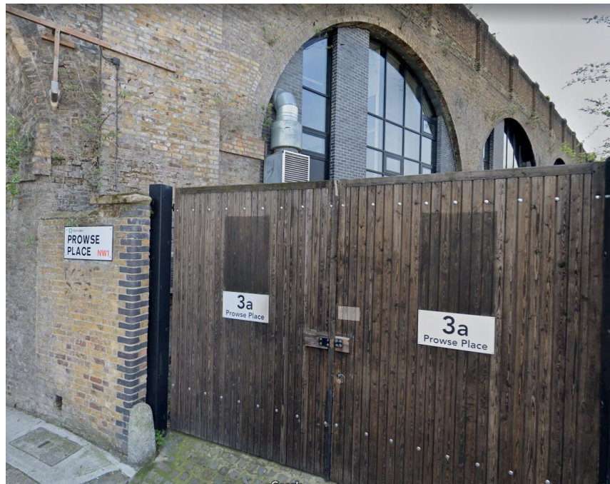
Figure 5.1: Existing Air Handling Units
