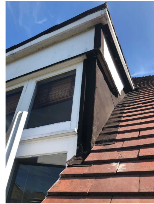
Side view of existing condition of flat roof dormer set within hip red tile roof.
