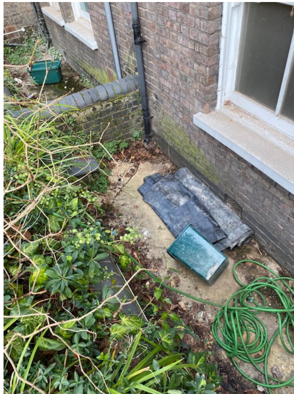
RWP 9 DISCHARGES ONTO GROUND
