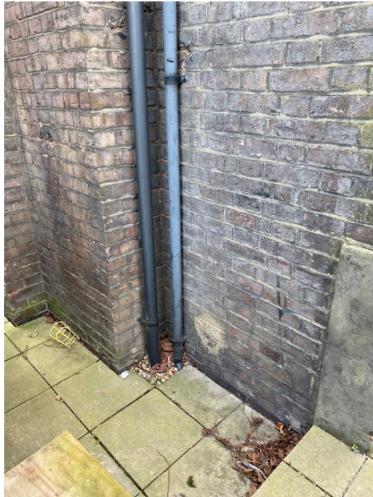
RWP'S 5 & 6: NO ACCESS
