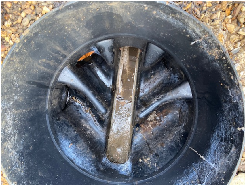
FW02: DEBRIS DEPOSITS
