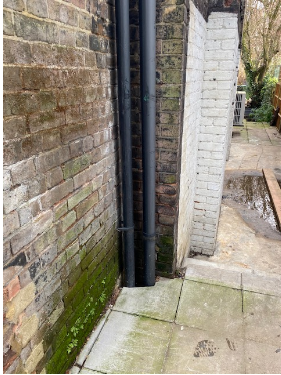
RWP 3 & 4: NO ACCESS
