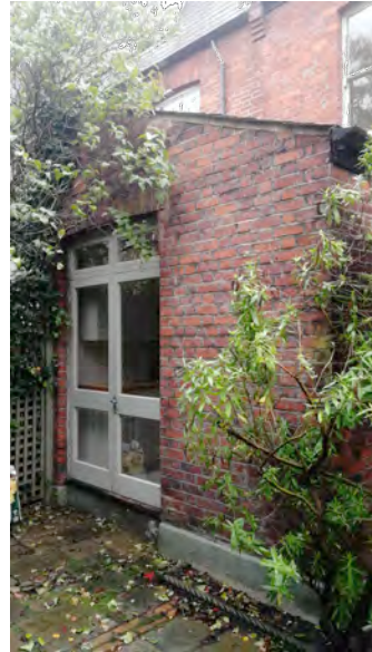
REAR FACADE OF KITCHEN PROJECTION: DOORS TO BE CONVERTED TO WINDOW WITH MATCHING APPEARANCE AND OPENING
