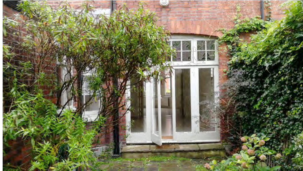
REAR FACADE OF MAIN HOUSE : FRENCH DOORS TO BE RECLAIMED AND RE-USED IN PROPOSED EXTENSION. PROPOSED 3m HIGH EXTENSION IS NO HIGHER THAN THE EXISTING FRENCH DOOR OPENING.
