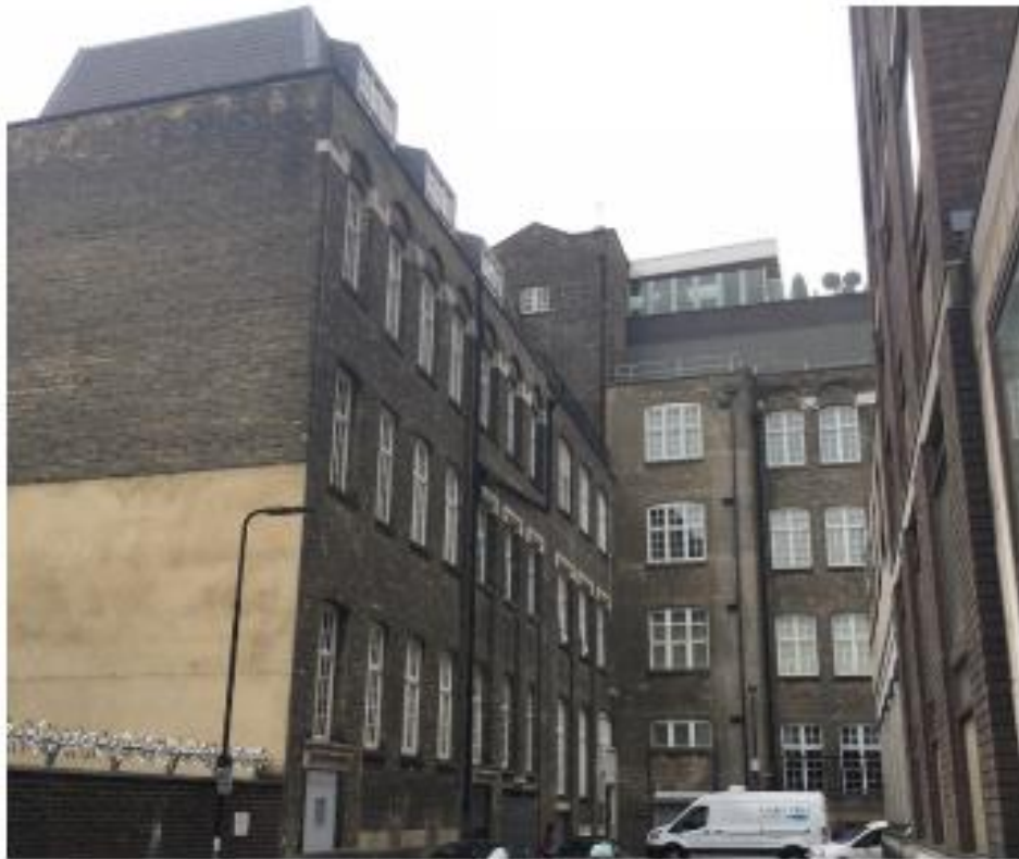
Rear north and east elevation of 30 Euston Square (taken from the north)
