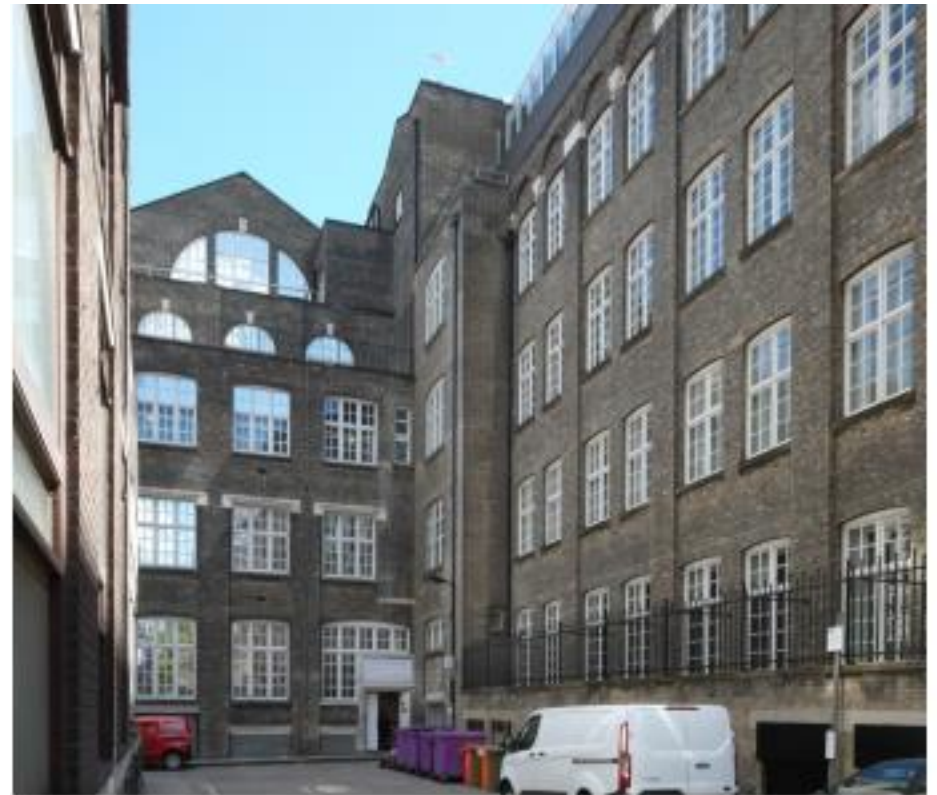
Rear north and east elevation of 30 Euston Square (taken from the east)
